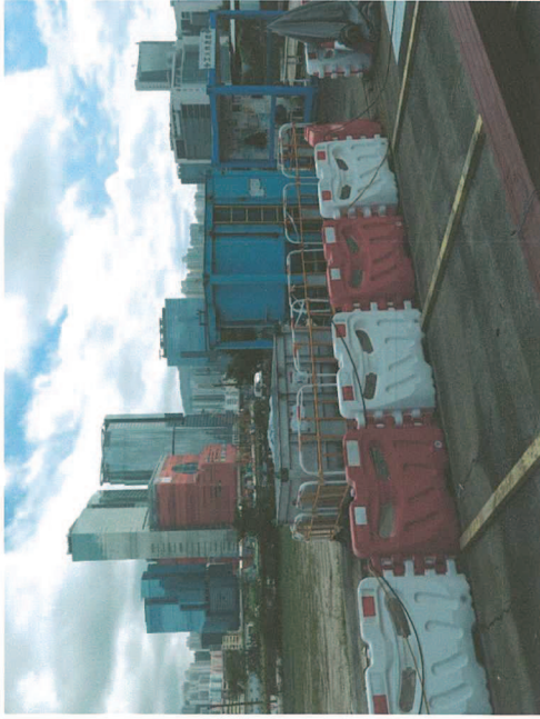
Wastewater Treatment Facility 廢水處理設施
