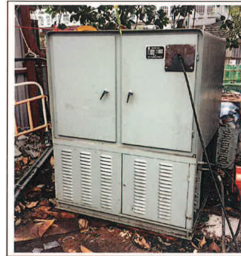
Power pack (diesel)
