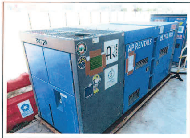
Generator, with Quality Powered Mechanical Equipment Label showing a Sound Power Level \leq 93 dB(A)
