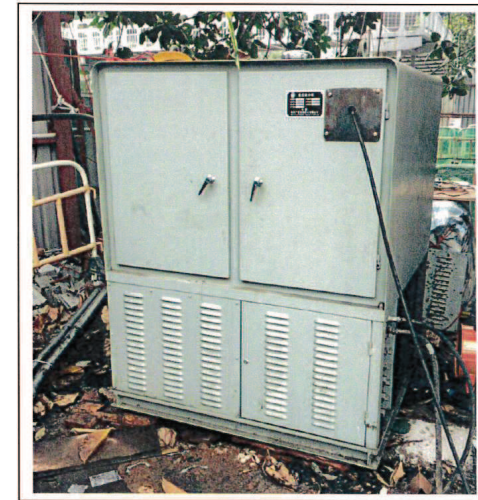
Power pack (diesel) 油渣動力供應器
