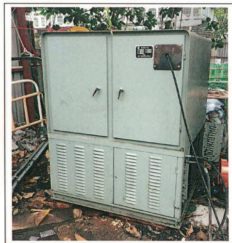
Power pack (diesel) 油渣動力供應器
