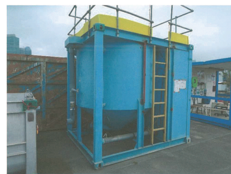
Wastewater Treatment Facility (2) 廢水處理設施(2)
