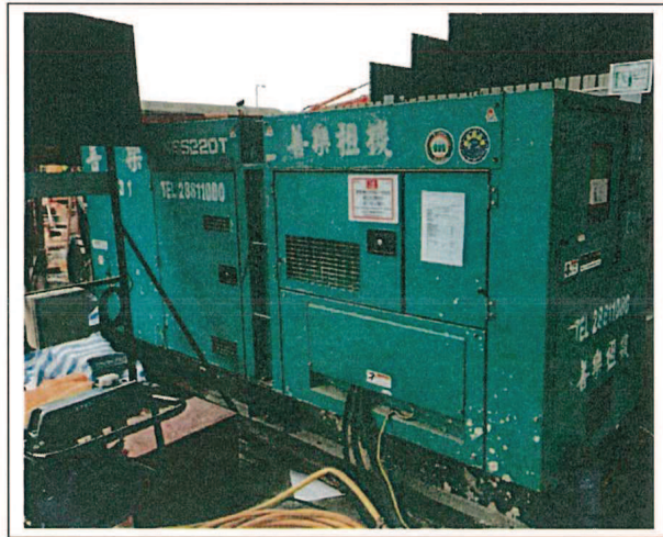
Generator, with Quality Powered Mechanical Equipment Label showing a Sound Power Level \leq 94\text{dB(A)} 發電機，備有優質機動設備標籤顯示聲功率級 \leq 94 分貝(A)
