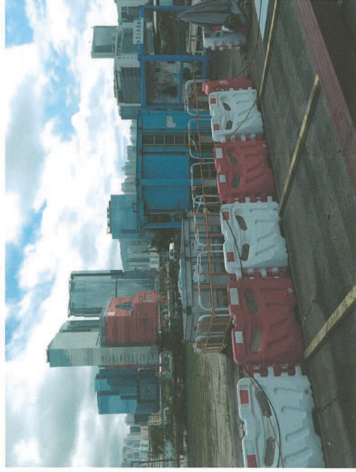
Wastewater Treatment Facility 廢水處理設施
