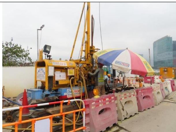
Lift LT1 & LT2 – ground investigation (DH17 & DH18), trial pit for locating underground utilities
