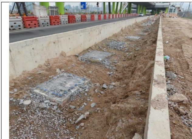
Noise Barriers – Breaking protection layer of the existing footings to expose the buried couplers, ground investigation (ADH6)
