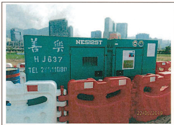
Generator, with Quality Powered Mechanical Equipment Label showing a Sound Power Level \leq 93 dB(A) 發電機，備有優質機動設備標籤顯示聲功率級 \leq 93 分貝(A)
