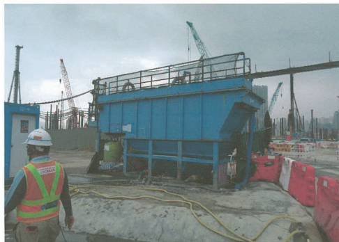
Wastewater Treatment Facility (1) 廢水處理設施(1)
