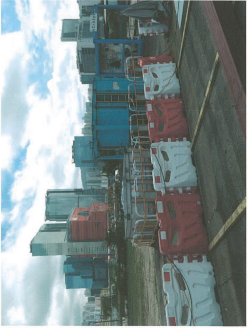
Wastewater Treatment Facility 廢水處理設施
