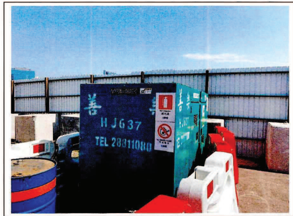
Generator, with Quality Powered Mechanical Equipment Label showing a Sound Power Level \leq 93 dB(A) (1) 發電機，備有優質機動設備標籤顯示聲功率級 \leq 93 分貝(A) (一)
