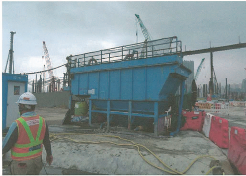
Wastewater Treatment Facility (1) 廢水處理設施(1)
