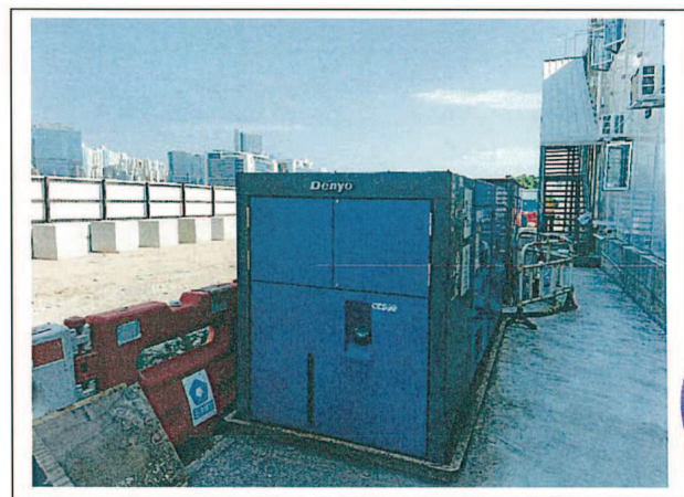
Generator, with Quality Powered Mechanical Equipment Label showing a Sound Power Level \leq 93 dB(A) 發電機，備有優質機動設備標籤顯示聲功率級 \leq 93 分貝(A)
