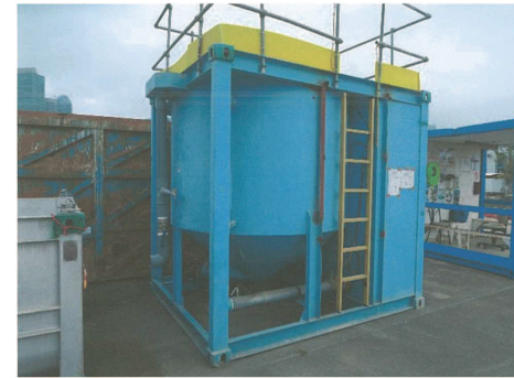
Wastewater Treatment Facility (2) 廢水處理設施(2)
