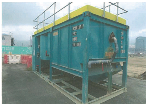
Wastewater Treatment Facility (3) 廢水處理設施(3)
