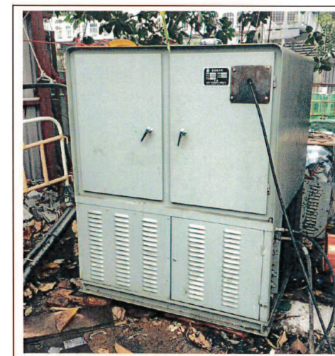
Power pack (diesel) 油渣動力供應器
