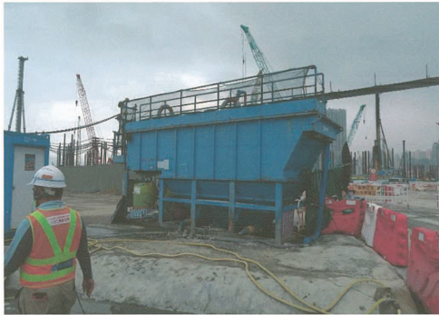
Wastewater Treatment Facility (1) 廢水處理設施(1)
