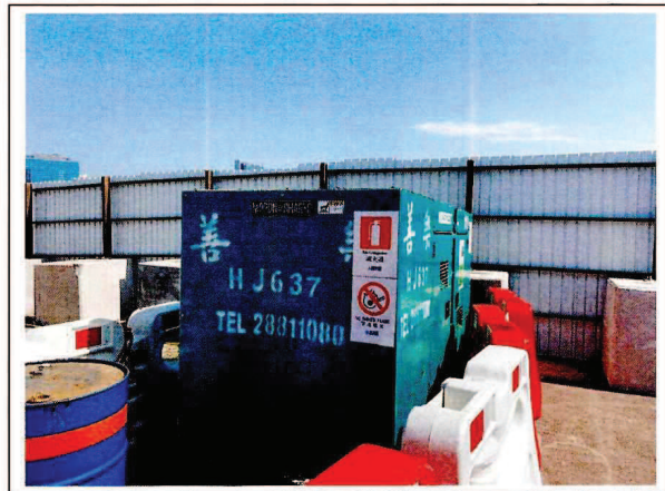
Generator, with Quality Powered Mechanical Equipment Label showing a Sound Power Level \leq 93 dB(A) (1) 發電機，備有優質機動設備標籤顯示聲功率級 \leq 93 分貝(A) (一)
