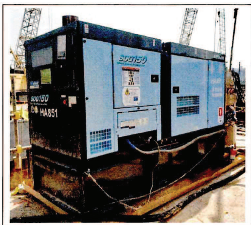
Generator, with Quality Powered Mechanical Equipment Label showing a Sound Power Level \leq 95 dB(A) 發電機，備有優質機動設備標籤顯示聲功率級 \leq 95 分貝(A)
