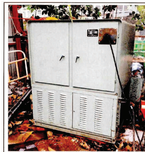
Power pack (diesel) 油渣動力供應器
