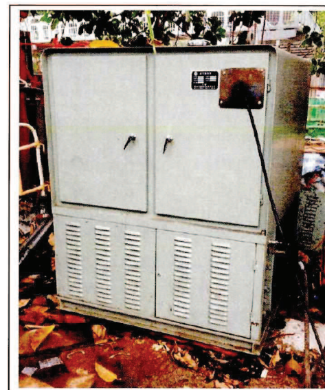
Power pack (diesel) 油渣動力供應器
