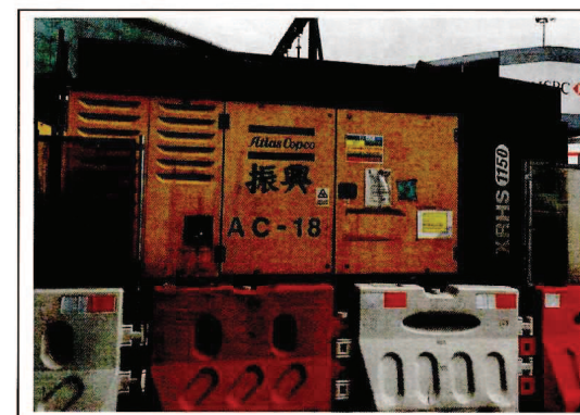
Air compressor, with Noise Emission Label showing a Sound Power Level of \leq 104 dB(A) 空氣壓縮機，備有噪音標籤顯示聲功率級 \leq 104 分貝(A)
