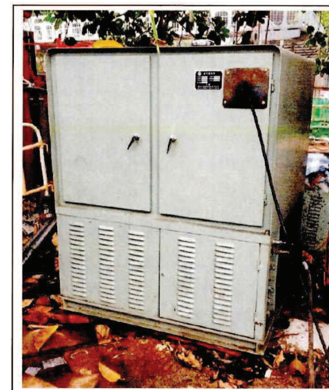
Power pack (diesel) 油渣動力供應器
