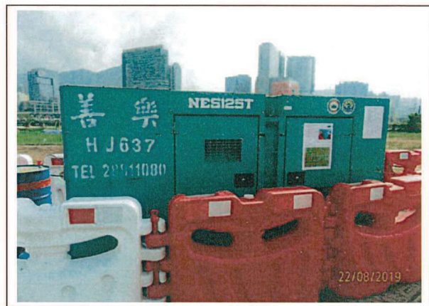
Generator, with Quality Powered Mechanical Equipment Label showing a Sound Power Level \leq 93 dB(A) 發電機，備有優質機動設備標籤顯示聲功率級 \leq 93 分貝(A)
