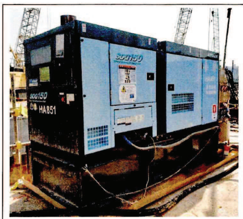
Generator, with Quality Powered Mechanical Equipment Label showing a Sound Power Level \leq 95 dB(A) 發電機，備有優質機動設備標籤顯示聲功率級 \leq 95 分貝(A)
