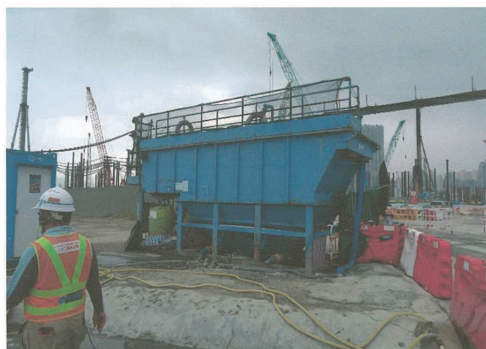
Wastewater Treatment Facility (1) 廢水處理設施(1)
