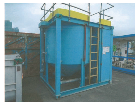
Wastewater Treatment Facility (2) 廢水處理設施(2)
