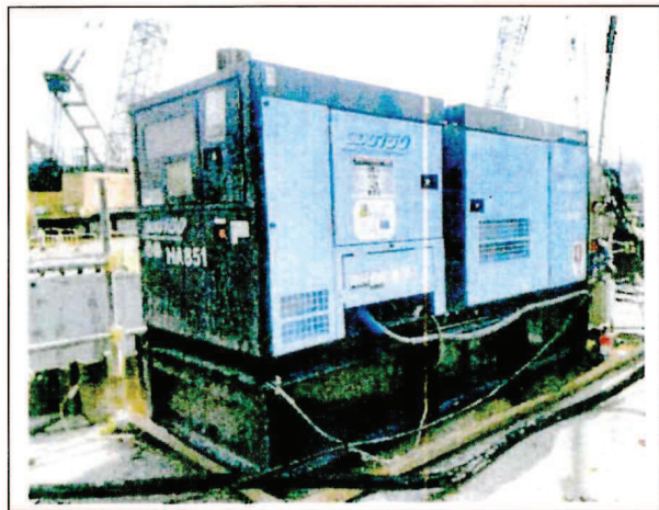
Generator, with Quality Powered Mechanical Equipment Label showing a Sound Power Level \leq 95\text{dB(A)} 發電機，備有優質機動設備標籤顯示聲功率級 \leq 95 分貝(A)
