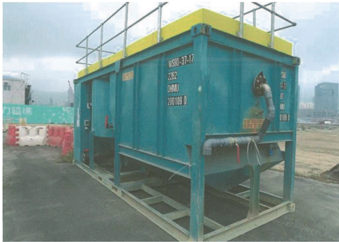
Wastewater Treatment Facility (3) 廢水處理設施(3)
