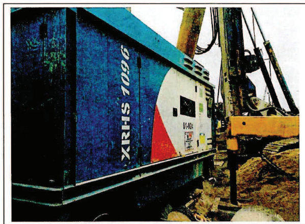
Air compressor, with Noise Emission Label showing a Sound Power Level of \leq 104\text{dB(A)} (2) 空氣壓縮機，備有噪音標籤顯示聲功率級 \leq 104 分貝(A) (二)
