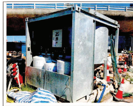
Wastewater treatment plant
