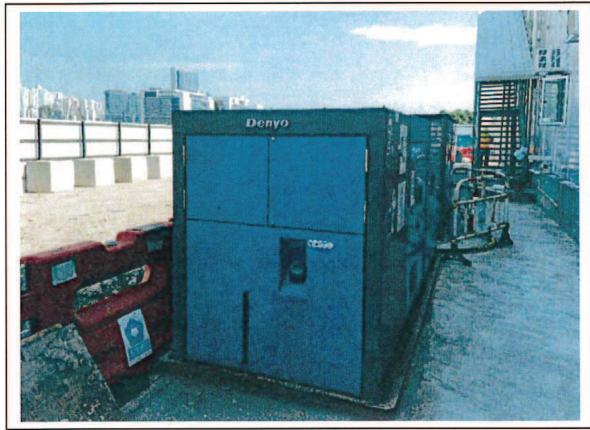
Generator, with Quality Powered Mechanical Equipment Label showing a Sound Power Level \leq 93 dB(A) 發電機，備有優質機動設備標籤顯示聲功率級 \leq 93 分貝(A)
