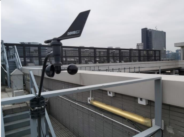
Weather Station at the rooftop of Hong Kong Children's Hospital
