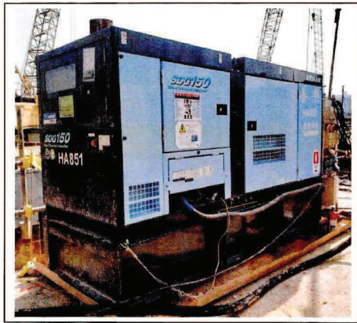
Generator, with Quality Powered Mechanical Equipment Label showing a Sound Power Level \leq 95 dB(A)
