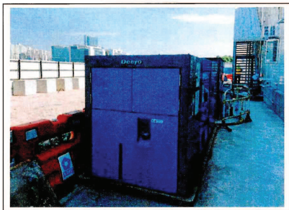
Generator, with Quality Powered Mechanical Equipment Label showing a Sound Power Level \leq 93 dB(A)
