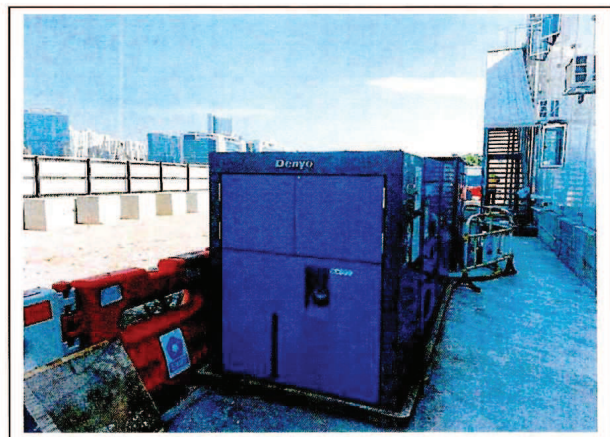
Generator, with Quality Powered Mechanical Equipment Label showing a Sound Power Level \leq 93 dB(A) (2) 發電機，備有優質機動設備標籤顯示聲功率級 \leq 93 分貝(A) (二)
