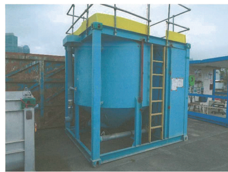
Wastewater Treatment Facility (2) 廢水處理設施(2)
