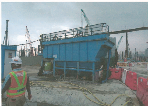
Wastewater Treatment Facility (1) 廢水處理設施(1)
