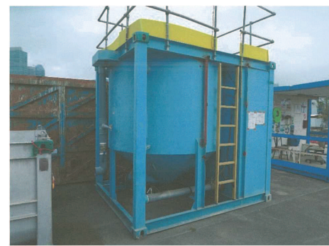
Wastewater Treatment Facility (2) 廢水處理設施(2)
