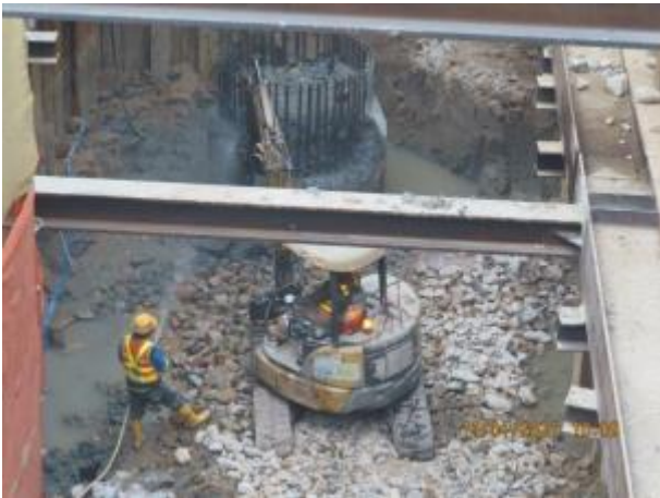
North Depressed Road – Construction of wall / dismantling of wailing & strut of cofferdam
