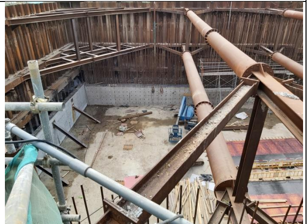
Construction of base slab and walls of Underpass and South Depressed Road
