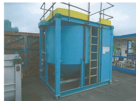
Wastewater Treatment Facility (2) 廢水處理設施(2)
