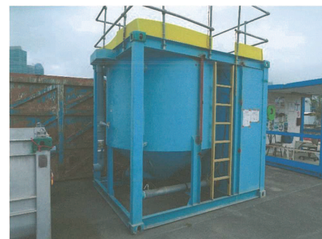
Wastewater Treatment Facility (2) 廢水處理設施(2)
