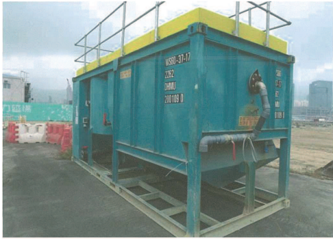
Wastewater Treatment Facility (3) 廢水處理設施(3)
