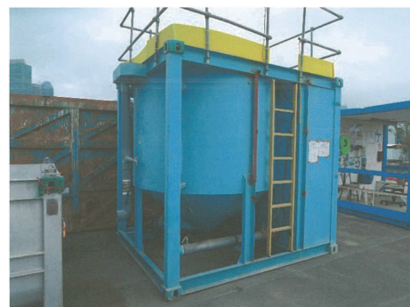
Wastewater Treatment Facility (2) 廢水處理設施(2)
