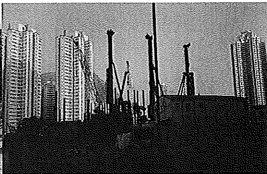
(Photo 2: Building construction site at the junction between Prince Edward Road East and King Kong Street)
