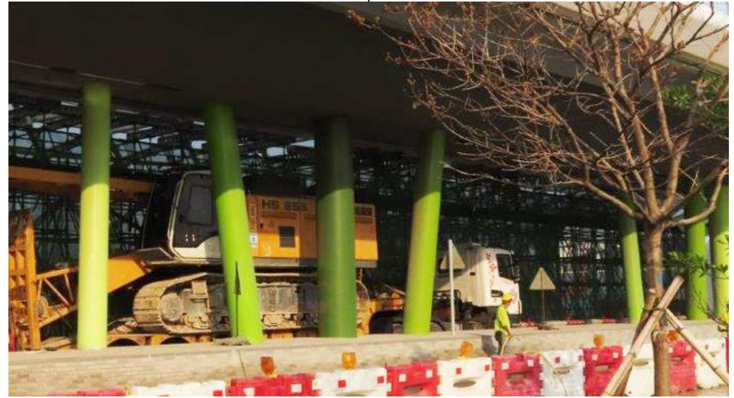
Reference photo of Elevated Landscaped Deck structure located at Kai Tak Stage 2 Development, column design to be echo and incorporated in this contract.
