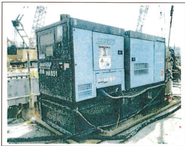
Generator, with Quality Powered Mechanical Equipment Label showing a Sound Power Level \leq 95\text{dB(A)} 發電機，備有優質機動設備標籤顯示聲功率級 \leq 95 分貝(A)
