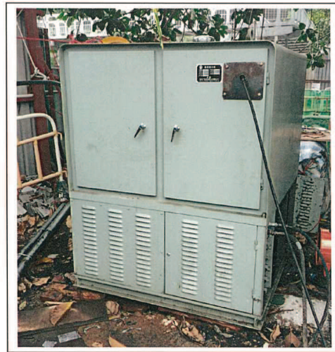
Power pack (diesel) 油渣動力供應器
