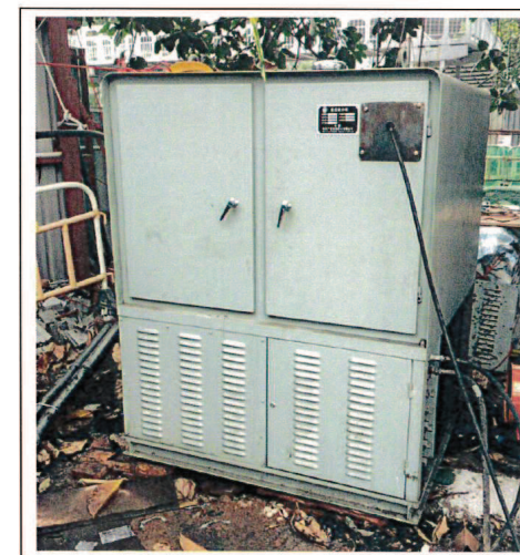
Power pack (diesel) 油渣動力供應器
