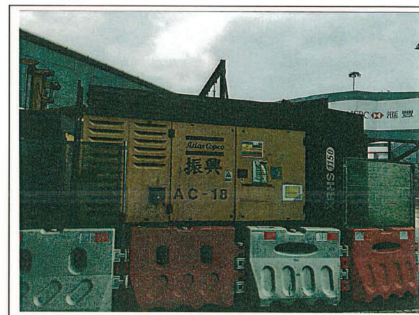
Air compressor, with Noise Emission Label showing a Sound Power Level of \leq 104 dB(A) (1) 空氣壓縮機，備有噪音標籤顯示聲功率級 \leq 104 分貝(A) (一)
