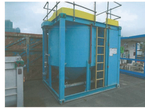
Wastewater Treatment Facility (2) 廢水處理設施(2)
