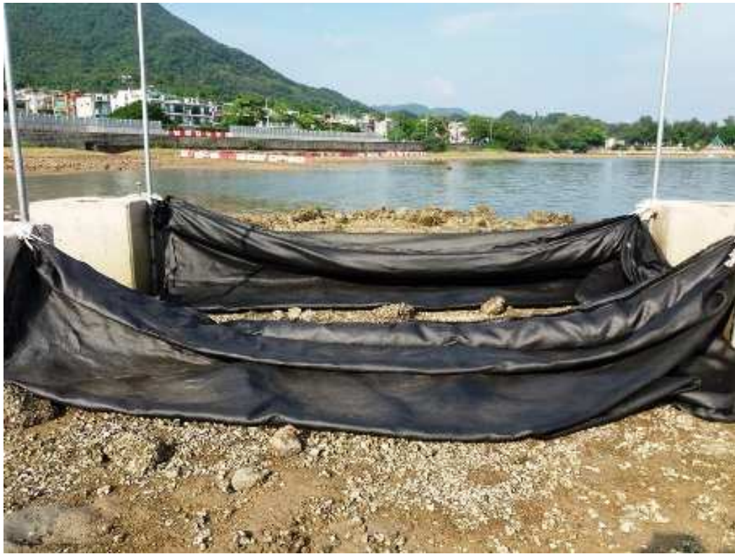
Photo 2. Demonstration of the fencing structure with concrete blocks and silt curtain on land
