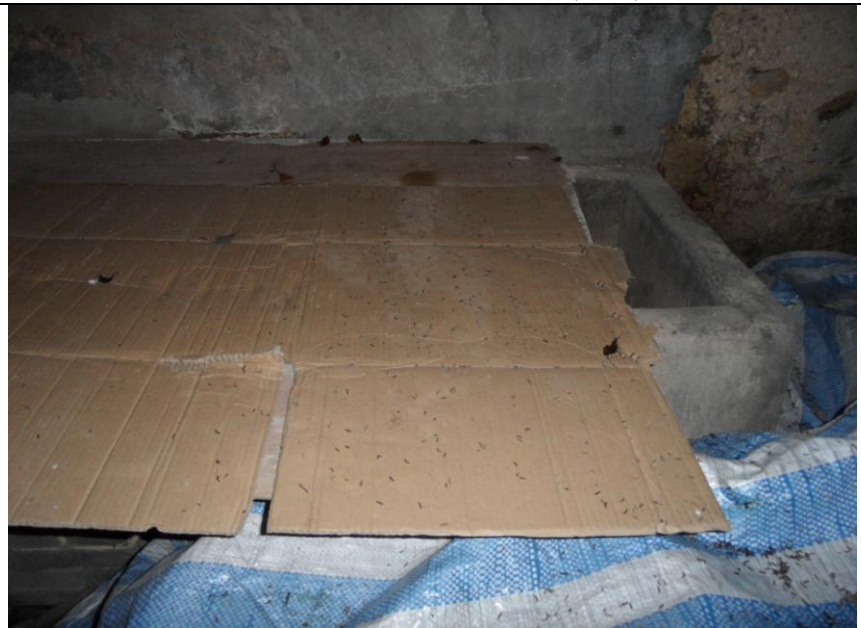
Kitchen Annex – Bat Faeces (27/9)
