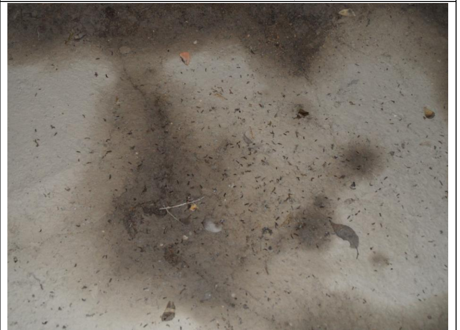
Kitchen Annex – Bat Faeces (27/10)
