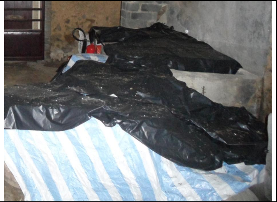
Kitchen Annex – Bat Faeces (01/11)
