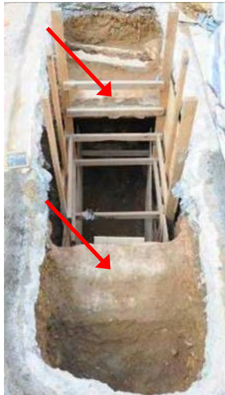
S1 in T2, with temporary wooden supporting system installed (view from south)
