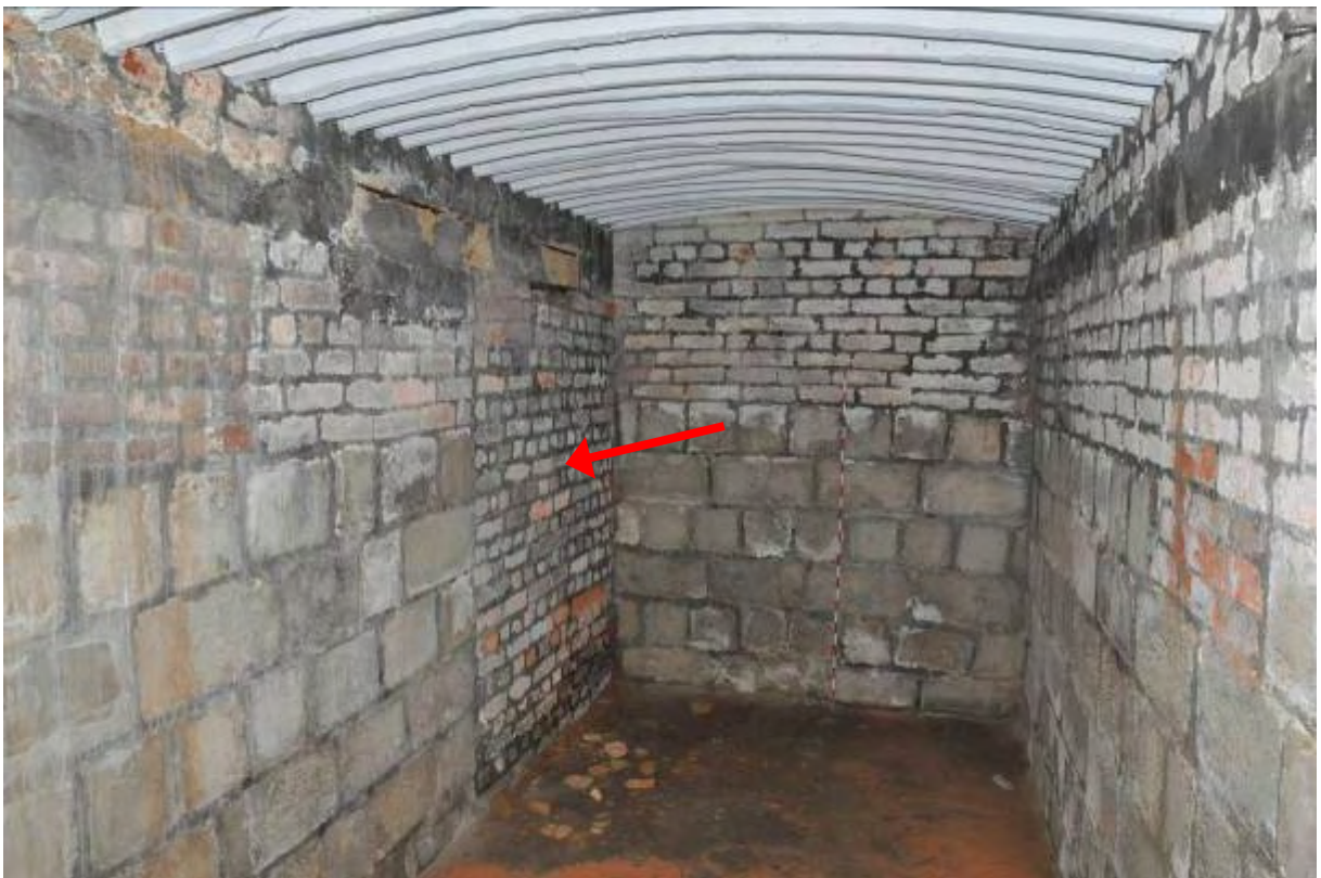
General view inside S12. The blocked entrance at the southern end east wall of S12 (view from north) leading to the passageway with steps (S2, S9)
