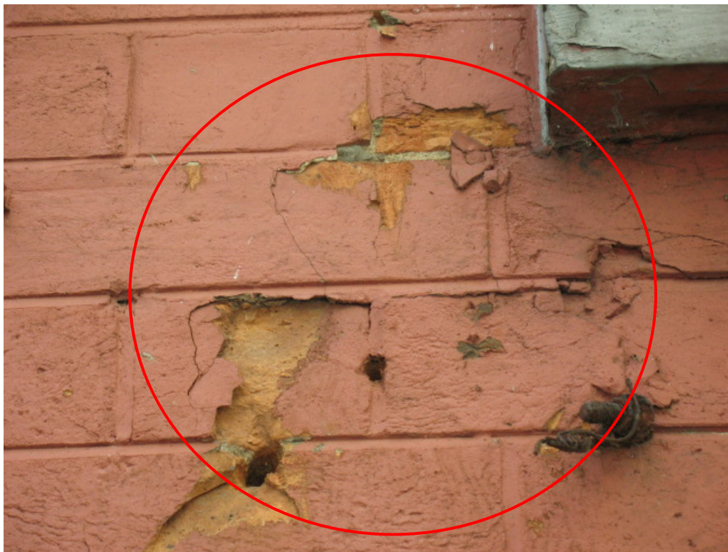
Photo ex 22e – The brickwork is damaged.
