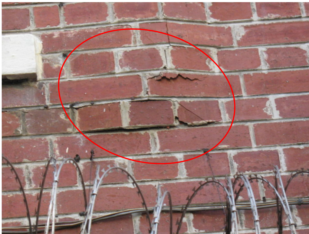
Photo ex 12b – The wall is damaged.
