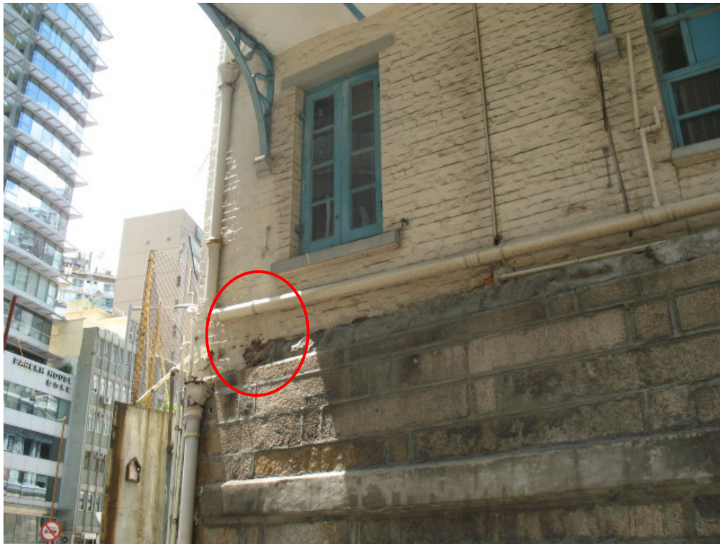
Photo ex 33a – The wall is damaged.
