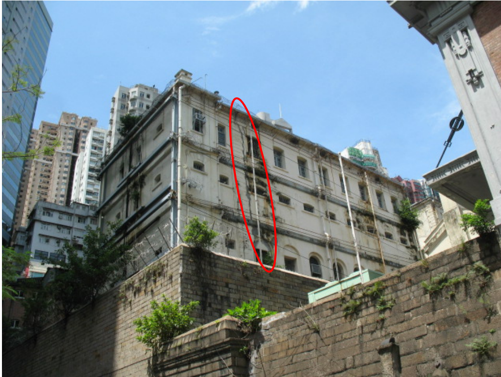
Photo ex 30a – Crack is found on the wall.
