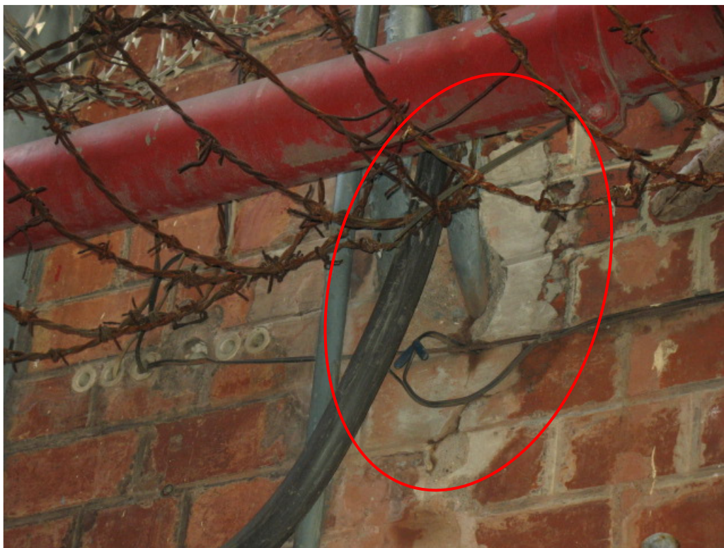
Photo ex 13b – The wall is damaged.
