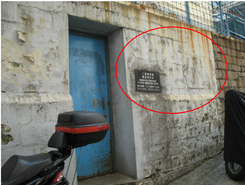
Photo ex 21a – Crack is found on the wall.
