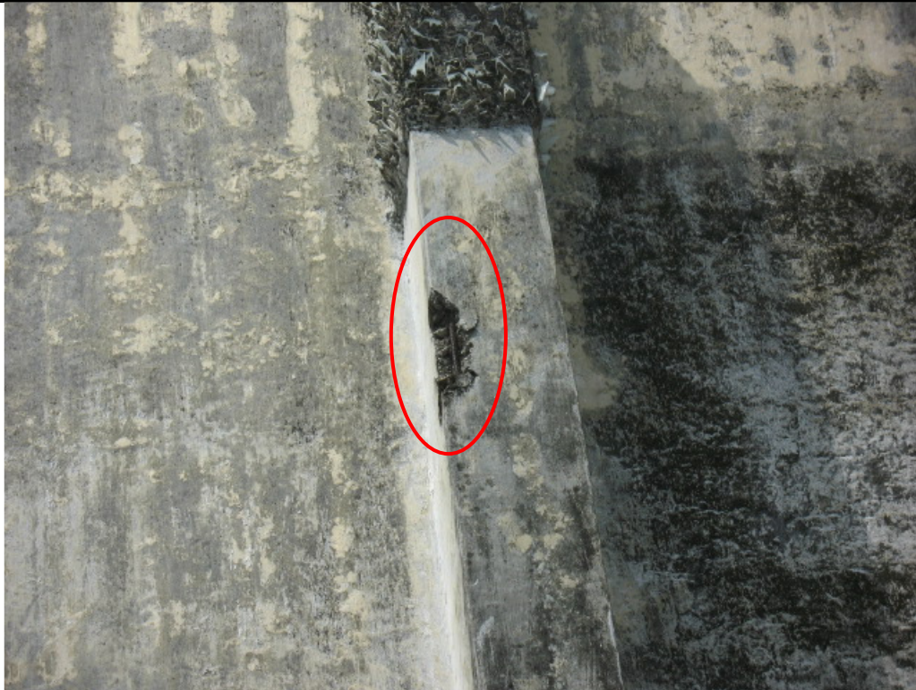
Photo ex 20b – The wall is damaged and steel bar is exposed.
