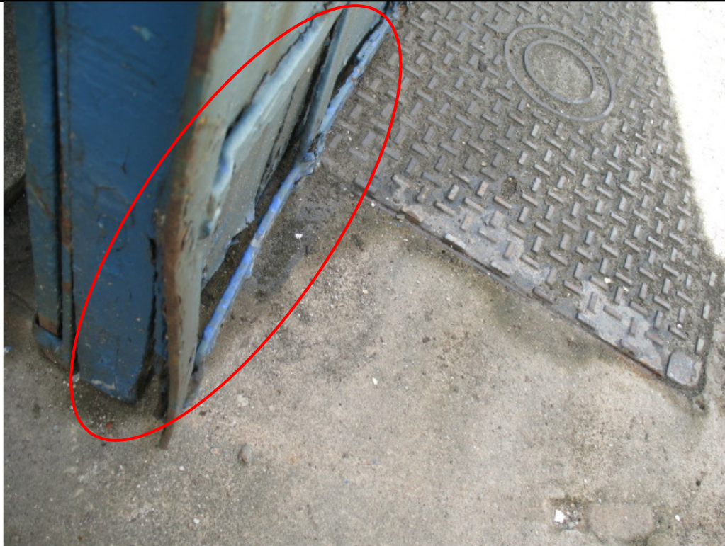
Photo ex 19b – Corrosion is found on the gate.
