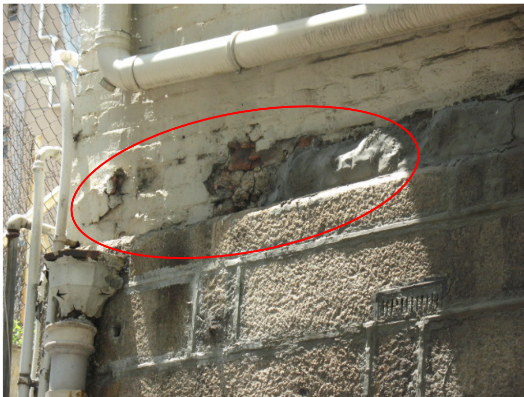
Photo ex 33b – The wall is damaged.
