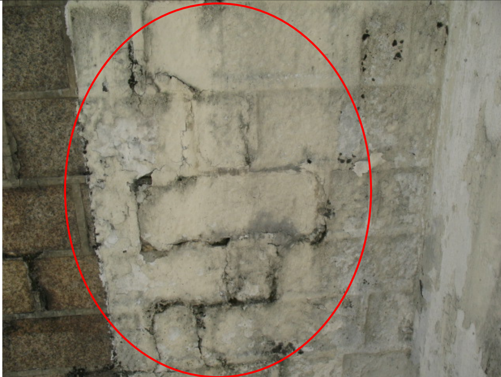
Photo ex 25b – Crack is found on the wall.
