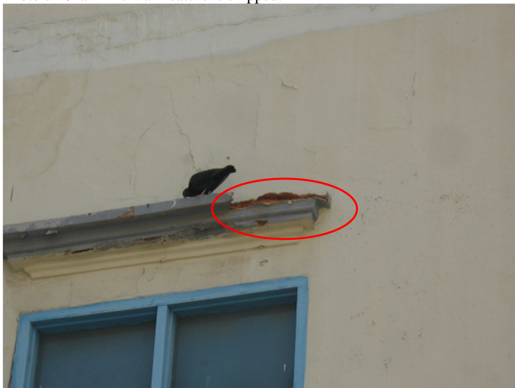
Photo ex 01b – The wall feature is chipped.
