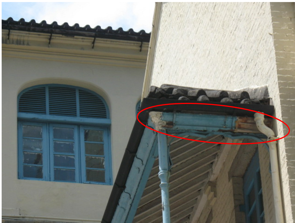
Photo ex 34b – The wooden balcony is damaged.
