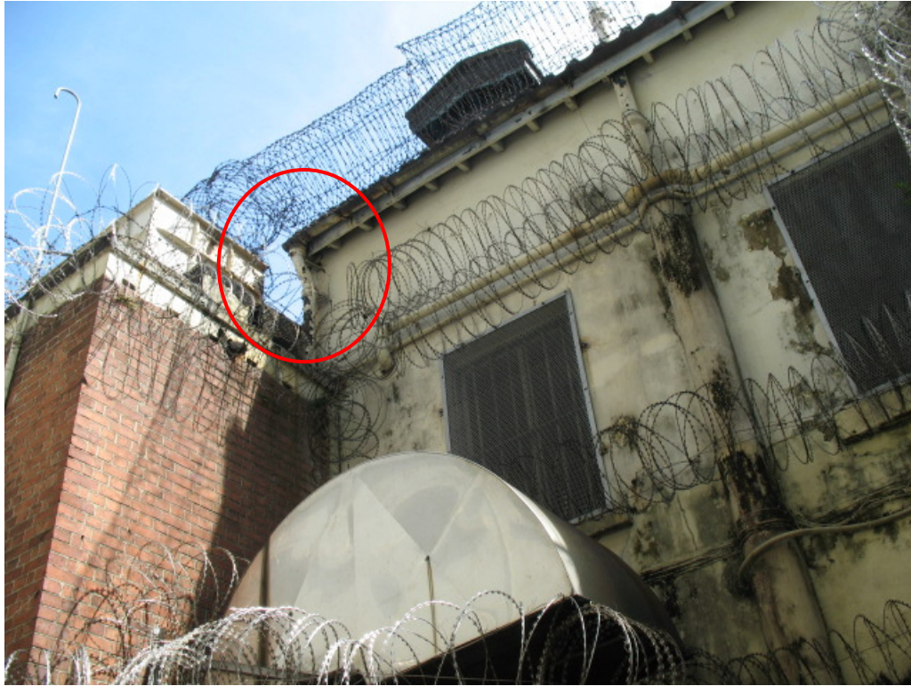
Photo ex 16a – Crack is found on the wall.
