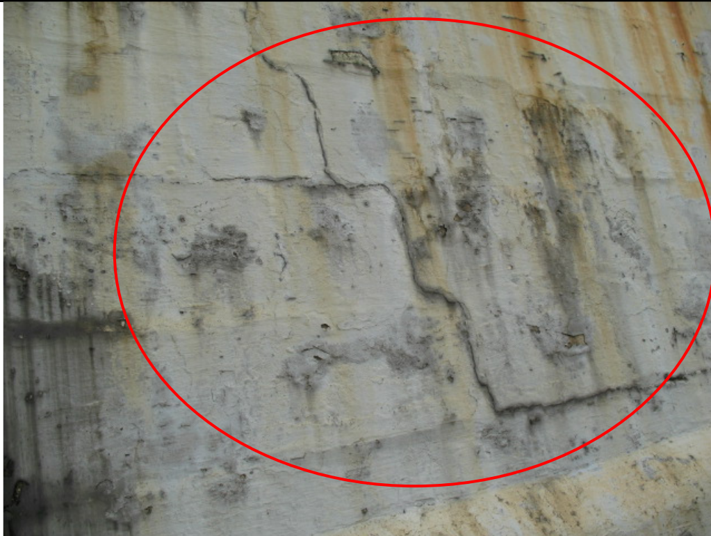
Photo ex 21b – Crack is found on the wall.
