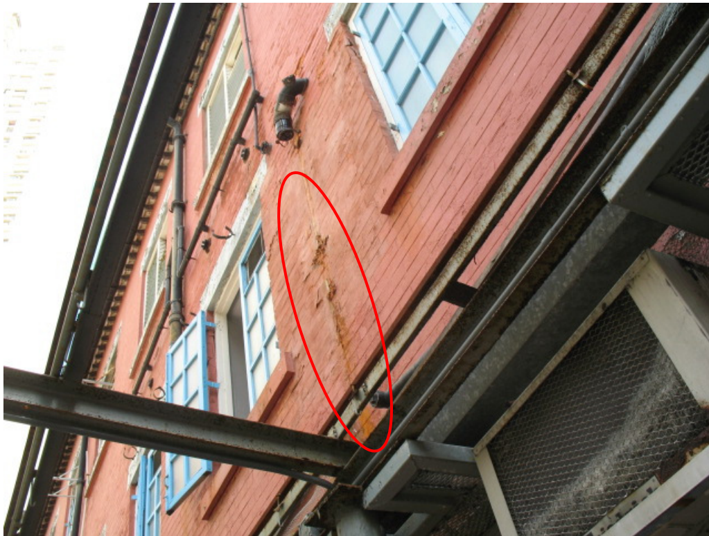
Photo ex 09a – The wall is damaged.
