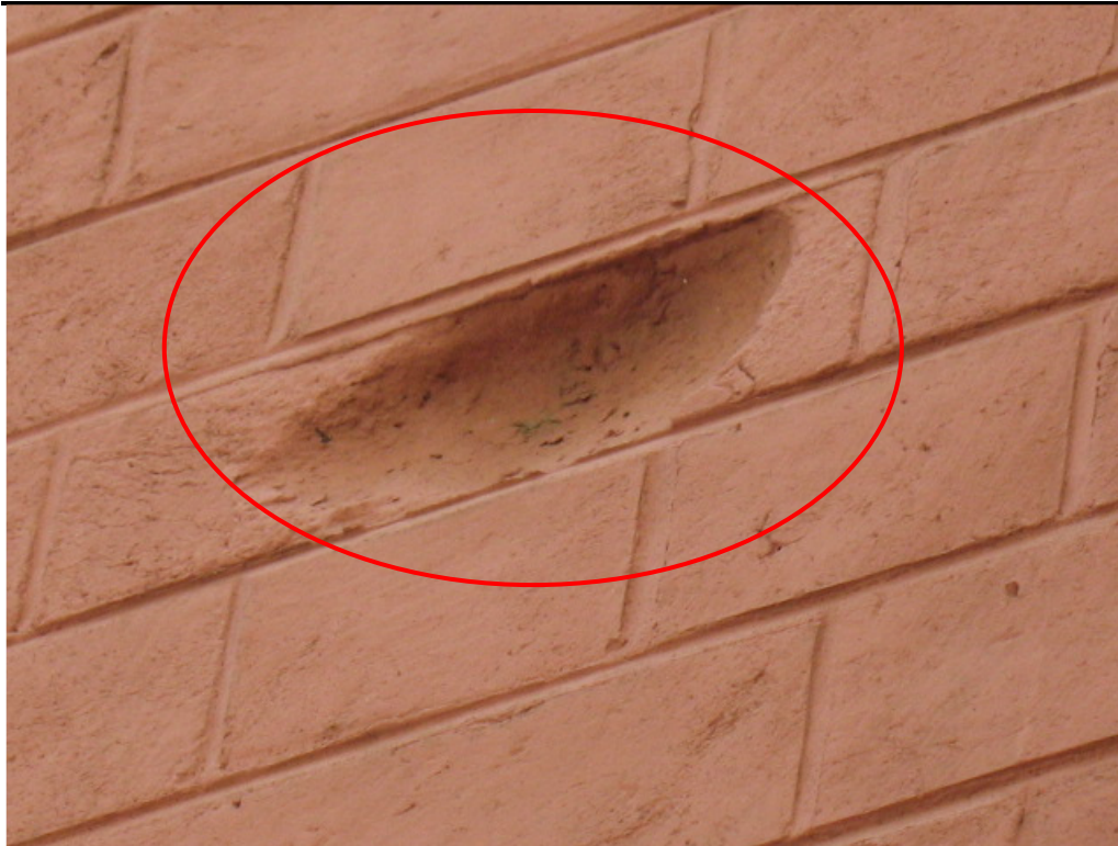
Photo ex 22d – The brick is chipped.
