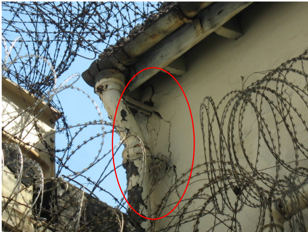
Photo ex 16b – Crack is found on the wall.
