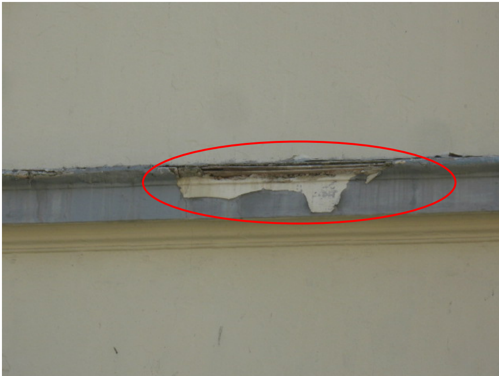
Photo ex 01d – The wall feature is damaged.
