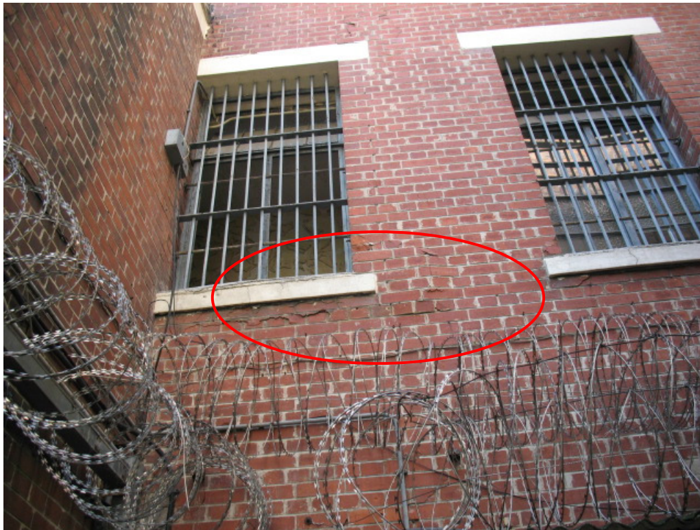
Photo ex 12a – The wall is damaged.
