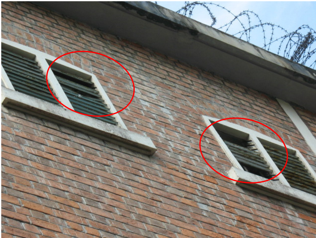
Photo ex 11c – The windows are damaged.
