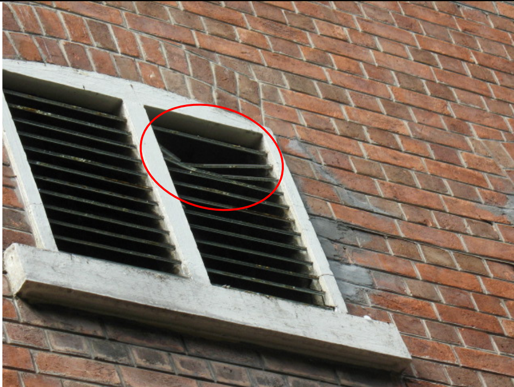
Photo ex 11b – The window is damaged.
