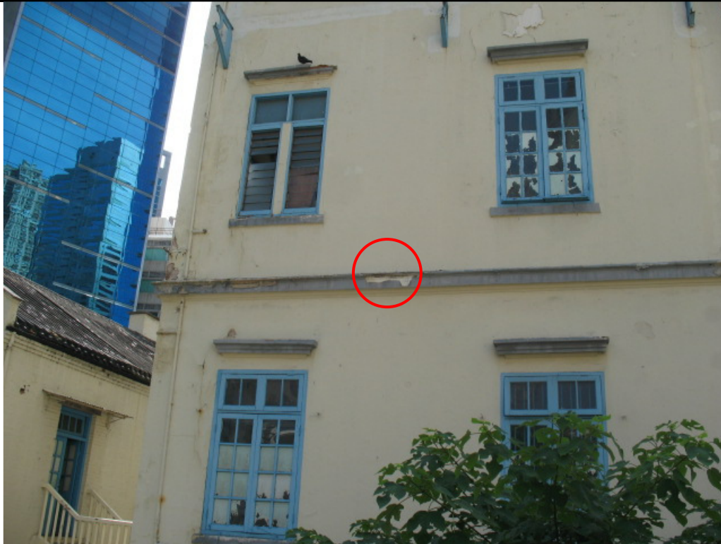
Photo ex 01c – The wall feature is damaged.
