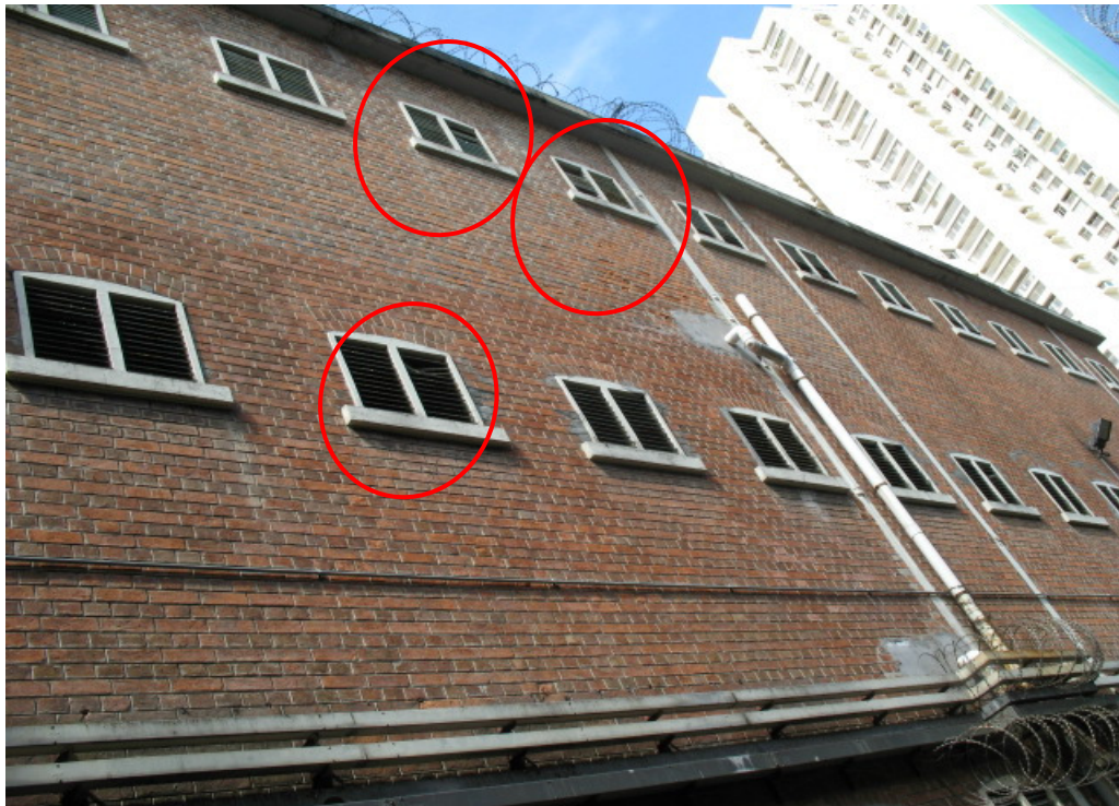
Photo ex 11a – The windows are damaged.
