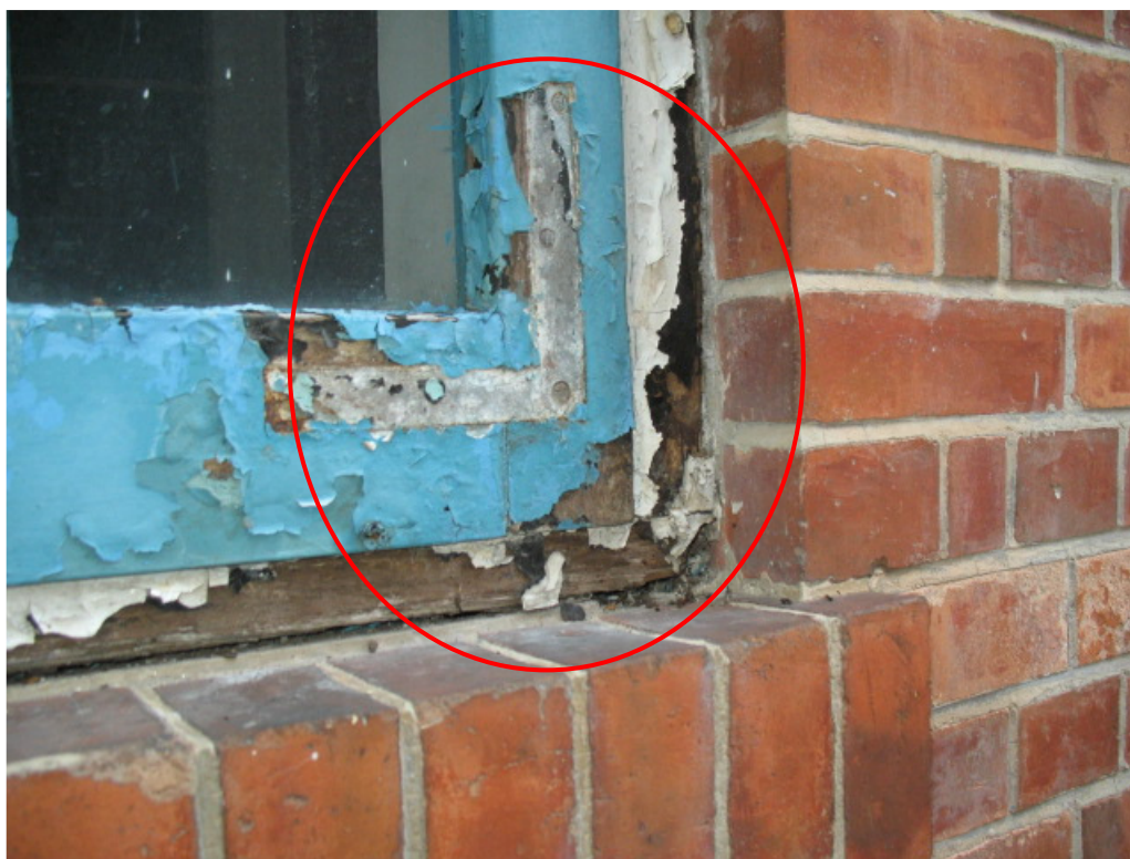
Photo ex 04b – The window frame is damaged.
