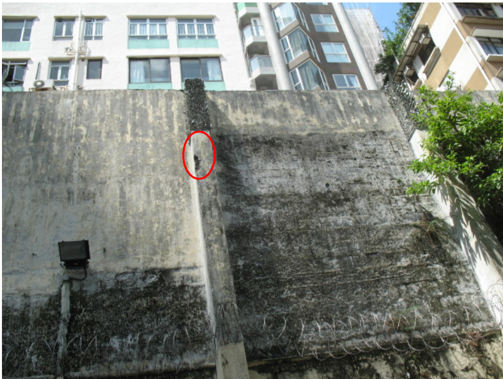
Photo ex 20a – The wall is damaged and steel bar is exposed.
