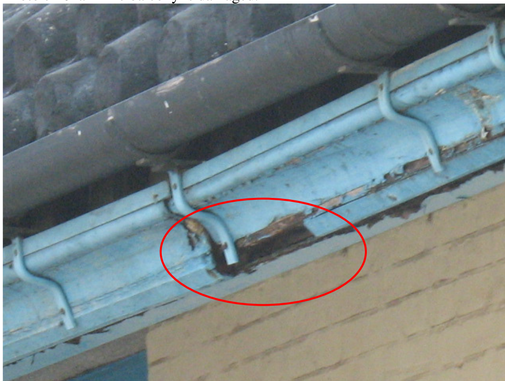
Photo ex 02b – The balcony is damaged.
