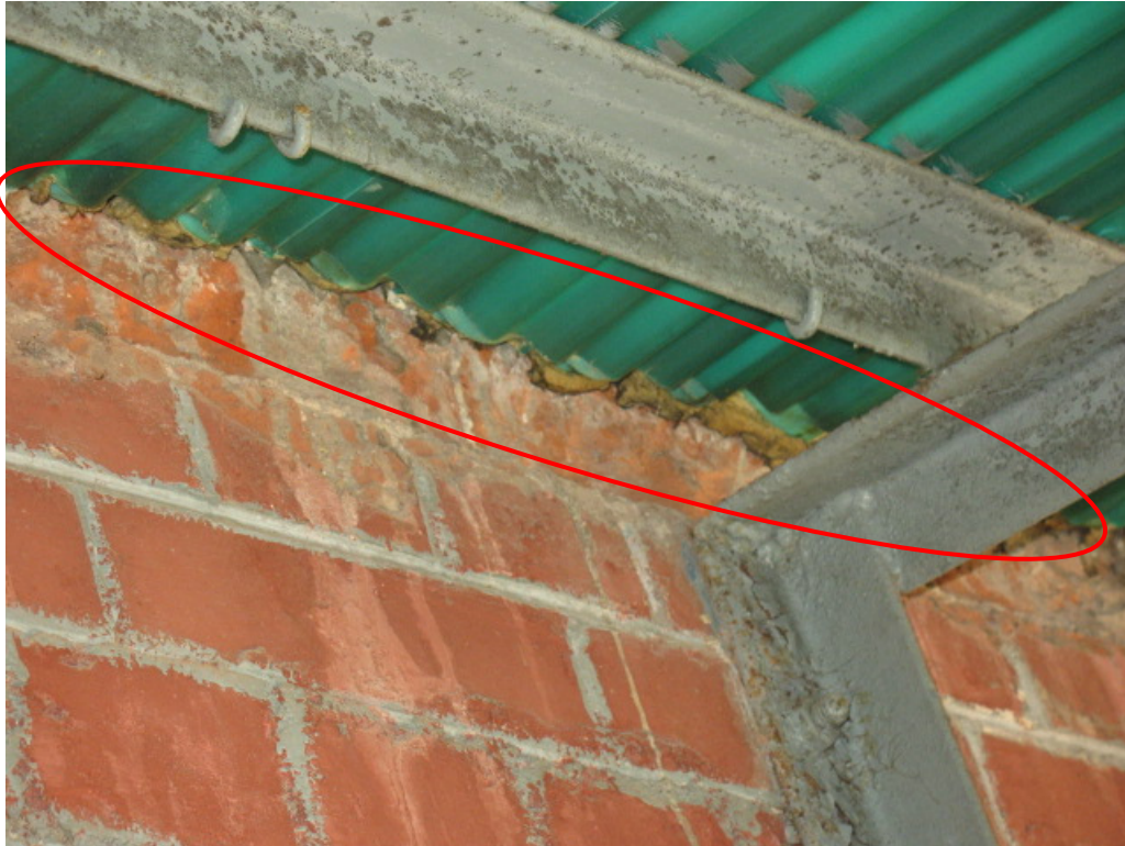
Photo ex 10a – The brickwork is chipped.
