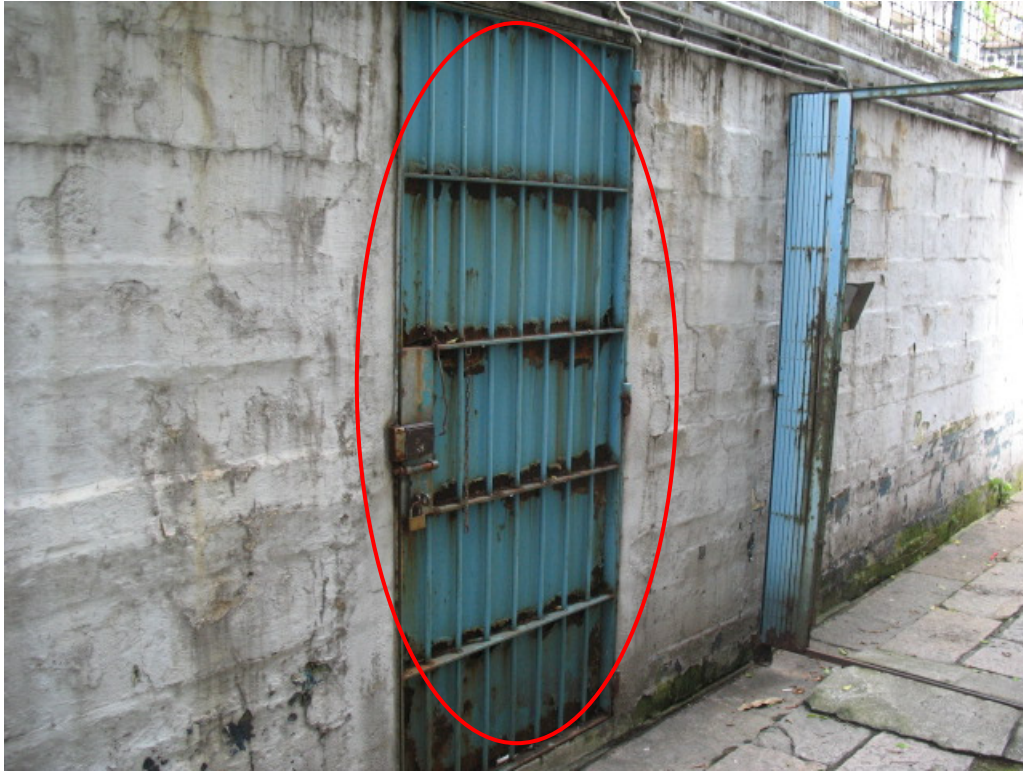
Photo ex 08a – Corrosion is found on the gate.
