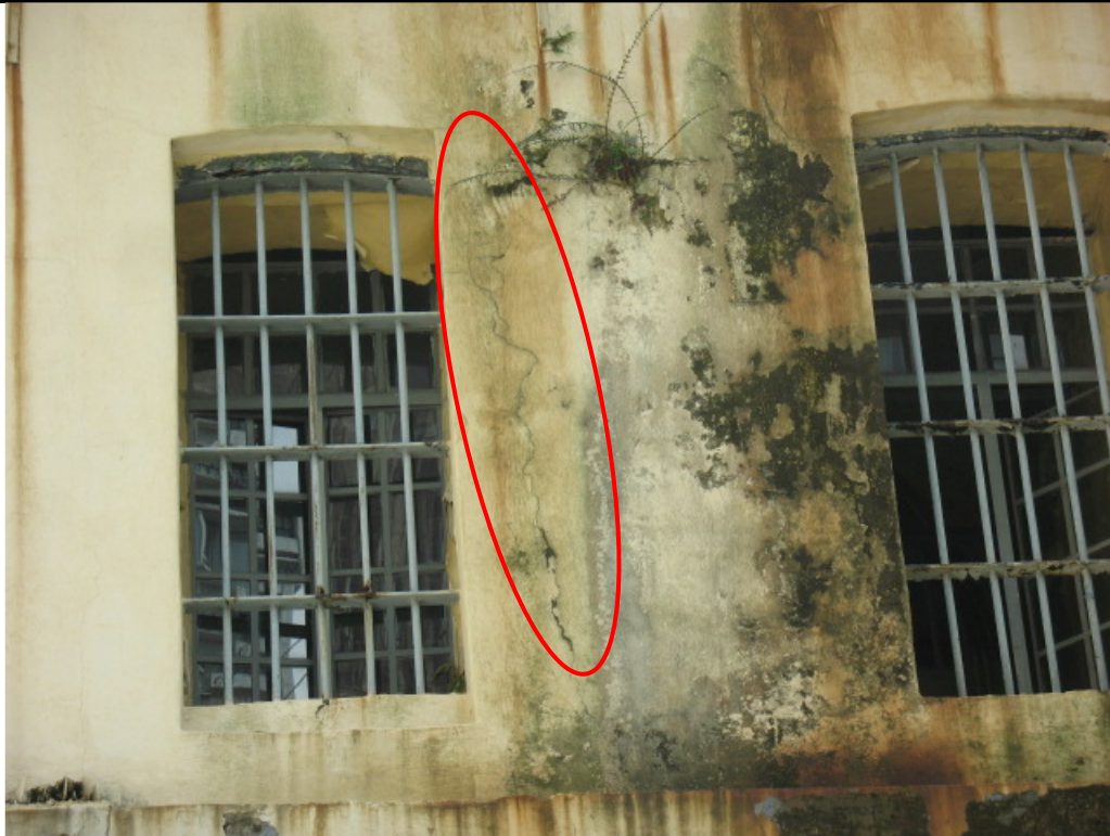
Photo ex 18b – Crack is found on the wall.
