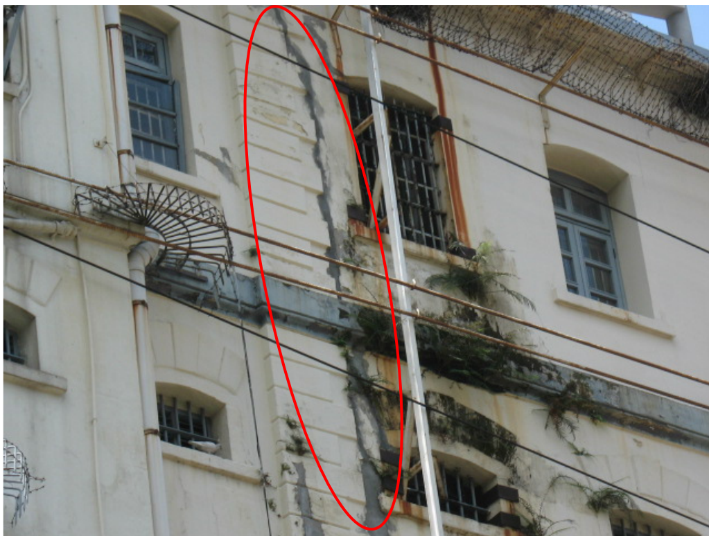
Photo ex 30b – Crack is found on the wall.
