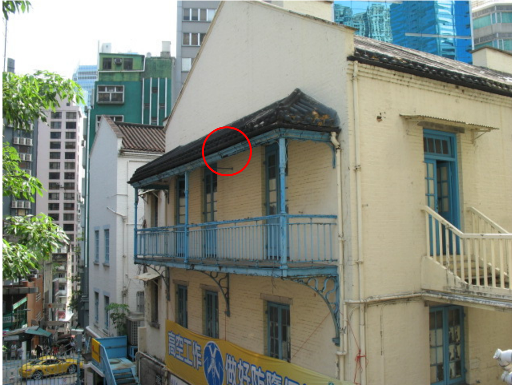
Photo ex 02a – The balcony is damaged.
