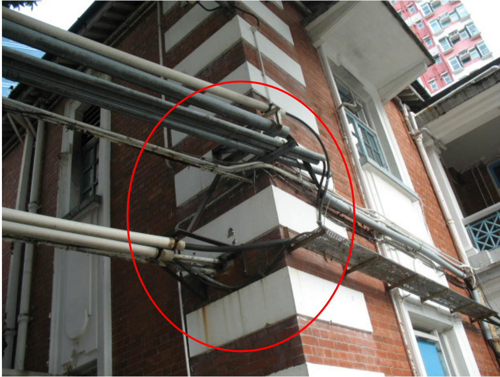
Photo ex 05a – The wall is damaged.
