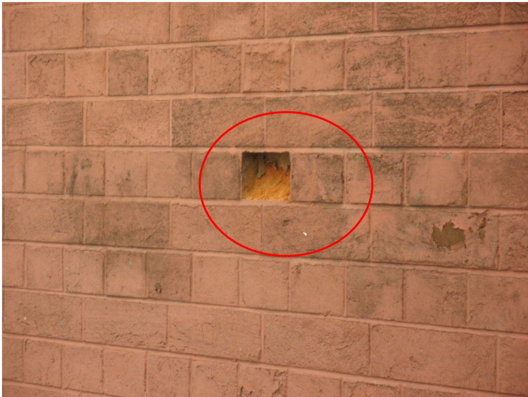
Photo ex 22c – The brickwork is damaged.
