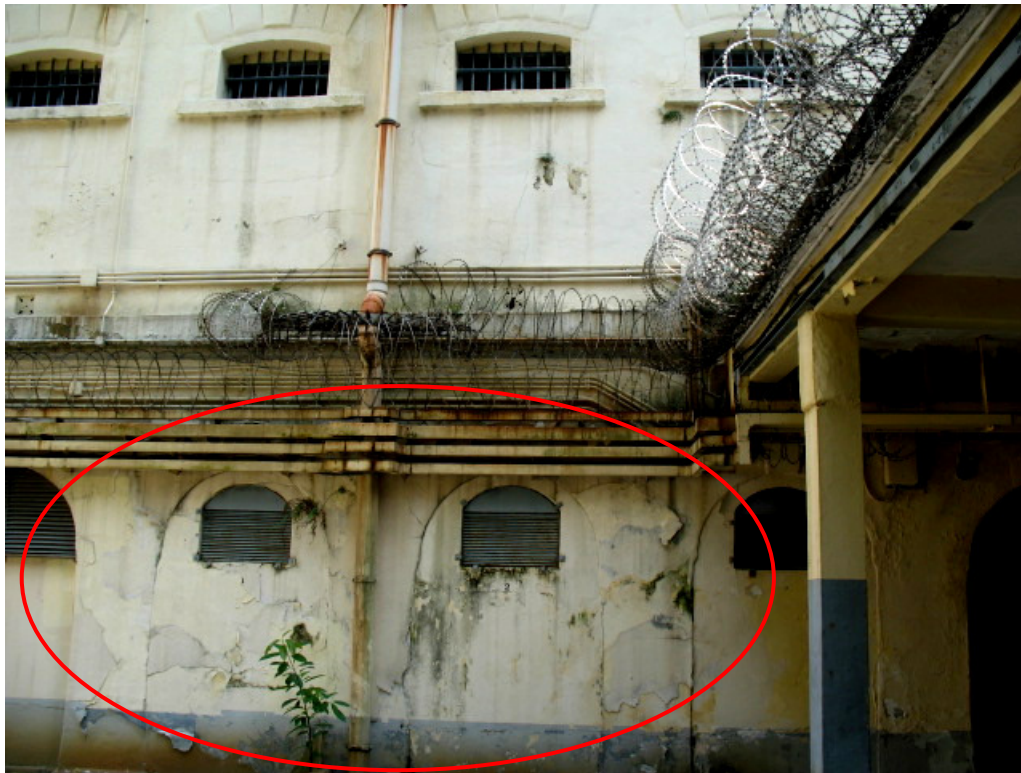
Photo ex 17a – Crack is found on the wall.
