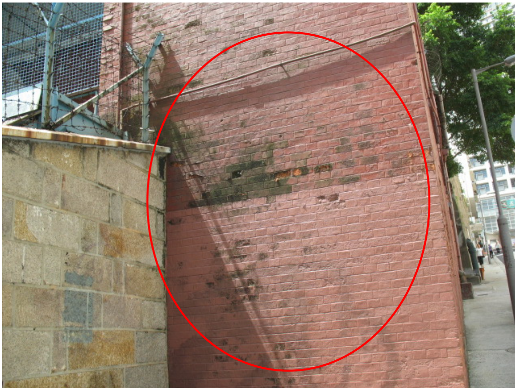
Photo ex 22a – The brick wall is damaged.
