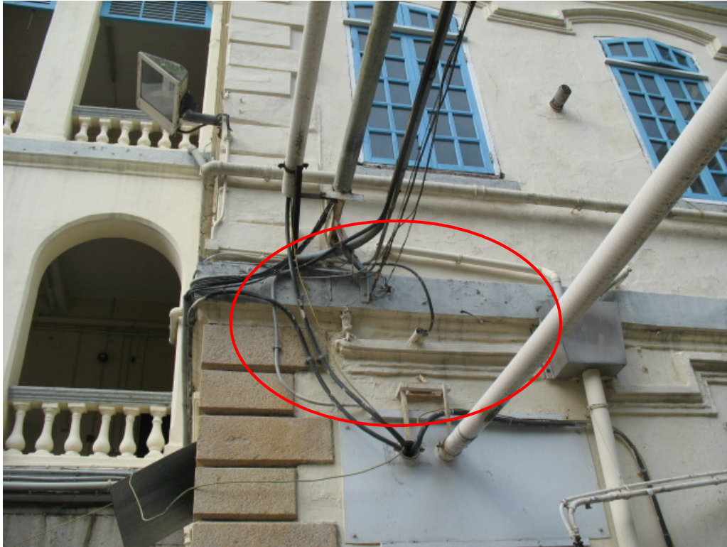
Photo ex 06a – The wall is damaged.
