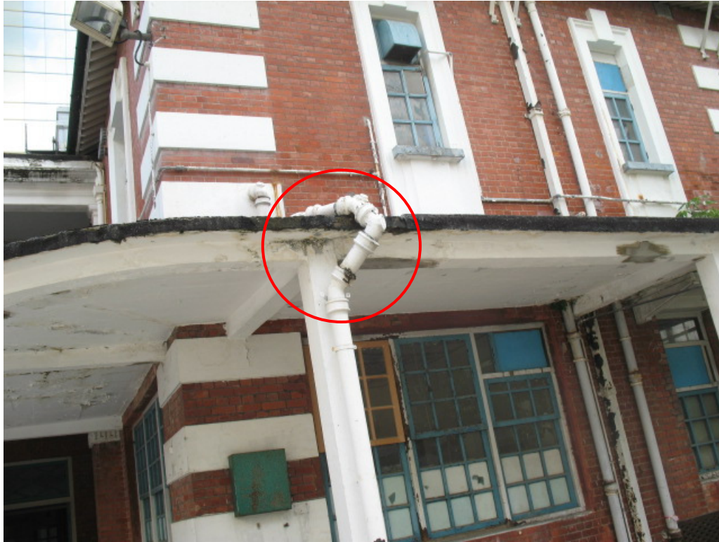
Photo ex 03a – Water stain is found is at the canopy.
