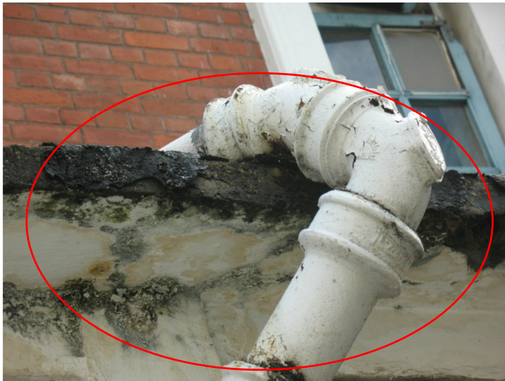
Photo ex 03b – Water stain is found at the canopy.
