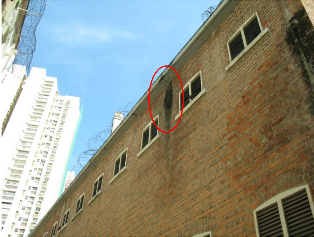
Photo ex 15a – Crack and water stain are found on the wall.
