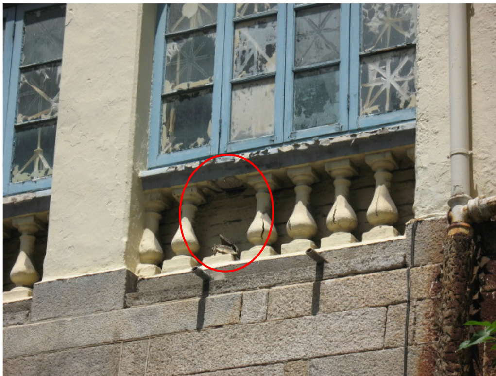
Photo ex 31b – One of the feature is missing.
