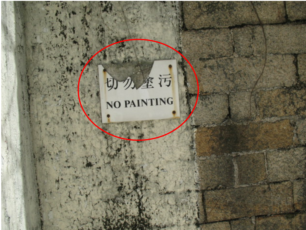
Photo ex 28a – The notice plaque is damaged.
