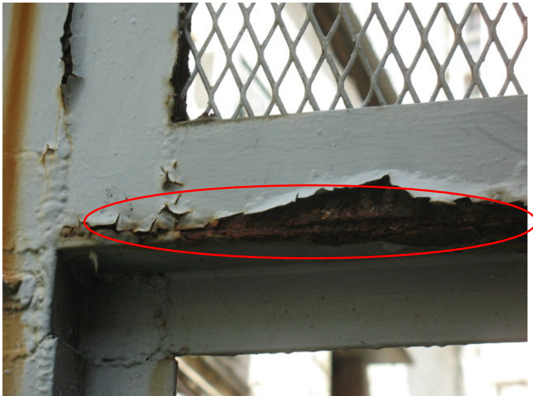
Photo ex 14b – Corrosion is found on the gate.
