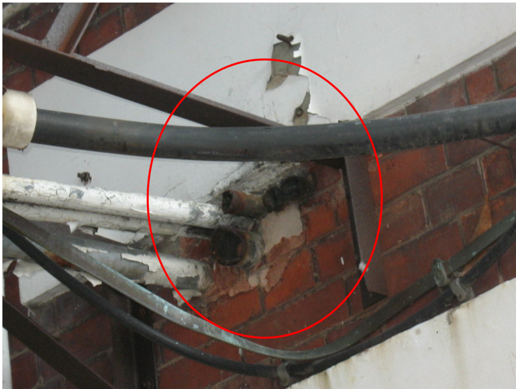
Photo ex 05b – The wall is damaged.
