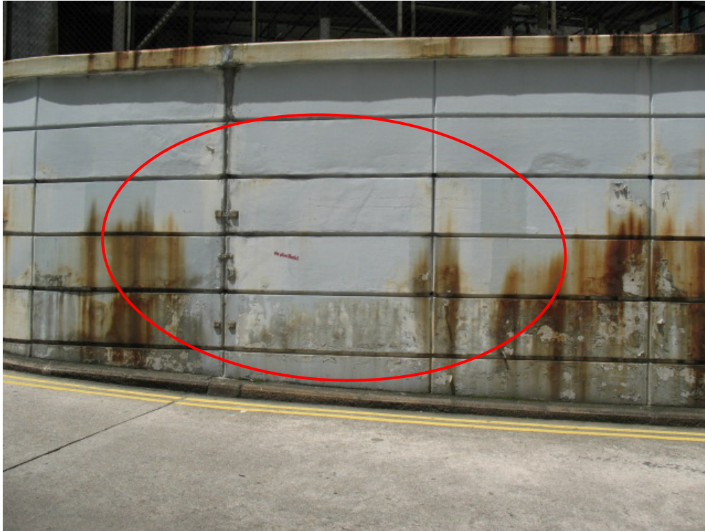
Photo ex 32a – Crack is found is found on the wall.
