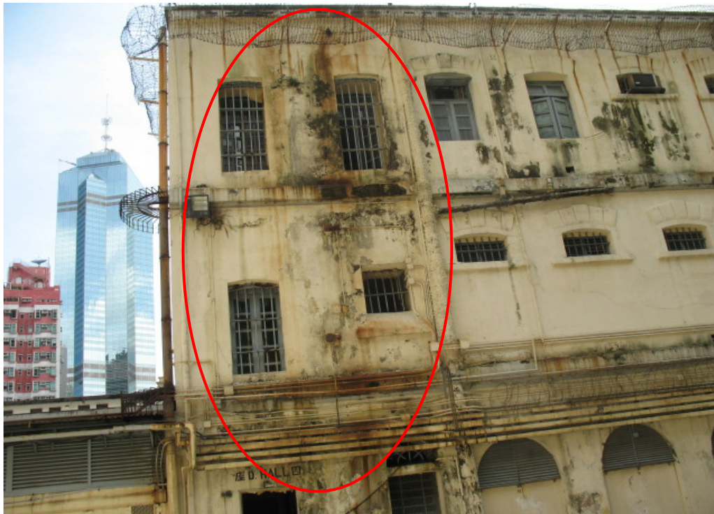
Photo ex 18a – Crack is found on the wall.
