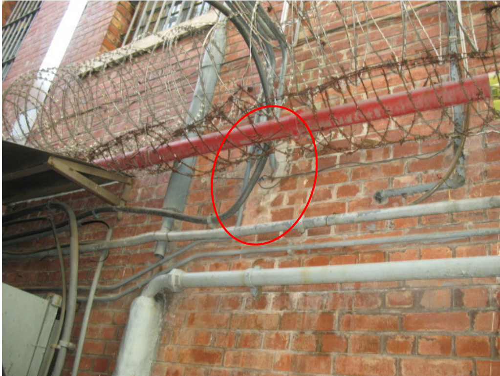
Photo ex 13a – The wall is damaged.
