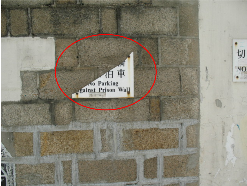
Photo ex 24a – The notice plaque is damaged.
