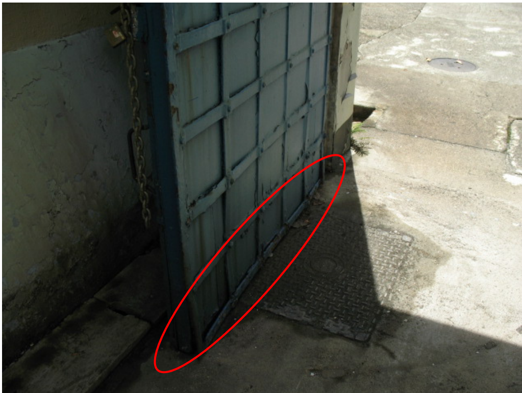
Photo ex 19a – Corrosion is found on the gate.
