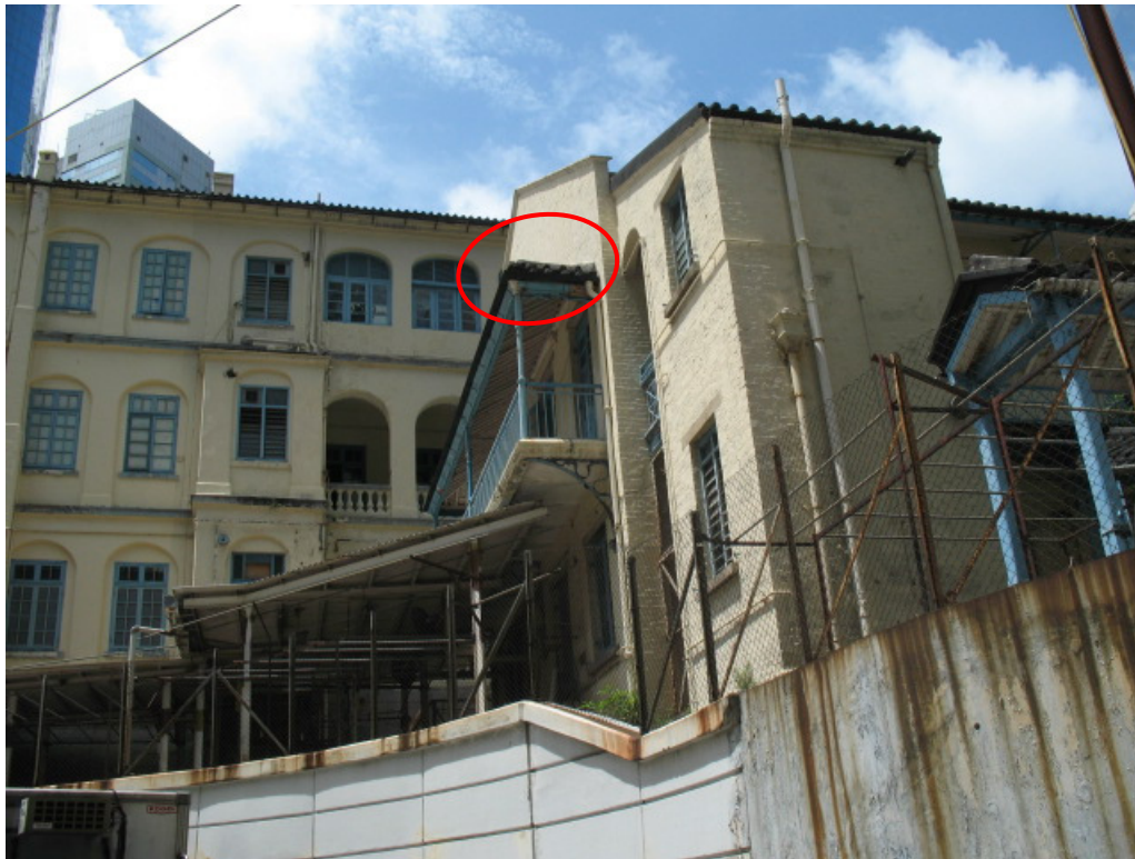
Photo ex 34a – The wooden balcony is damaged.
