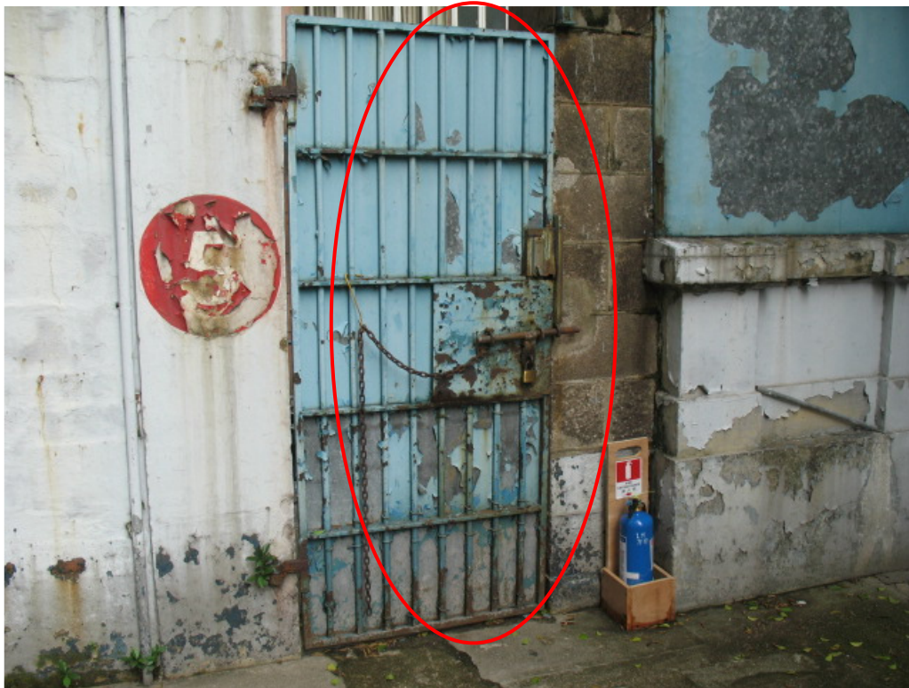
Photo ex 08b – Corrosion is found on the gate.
