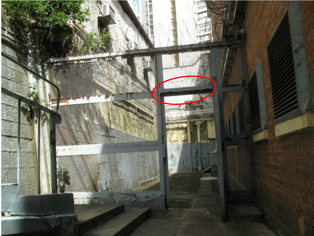
Photo ex 14a – Corrosion is found on the gate.
