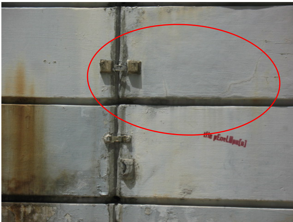
Photo ex 32b – Crack is found on the wall.
