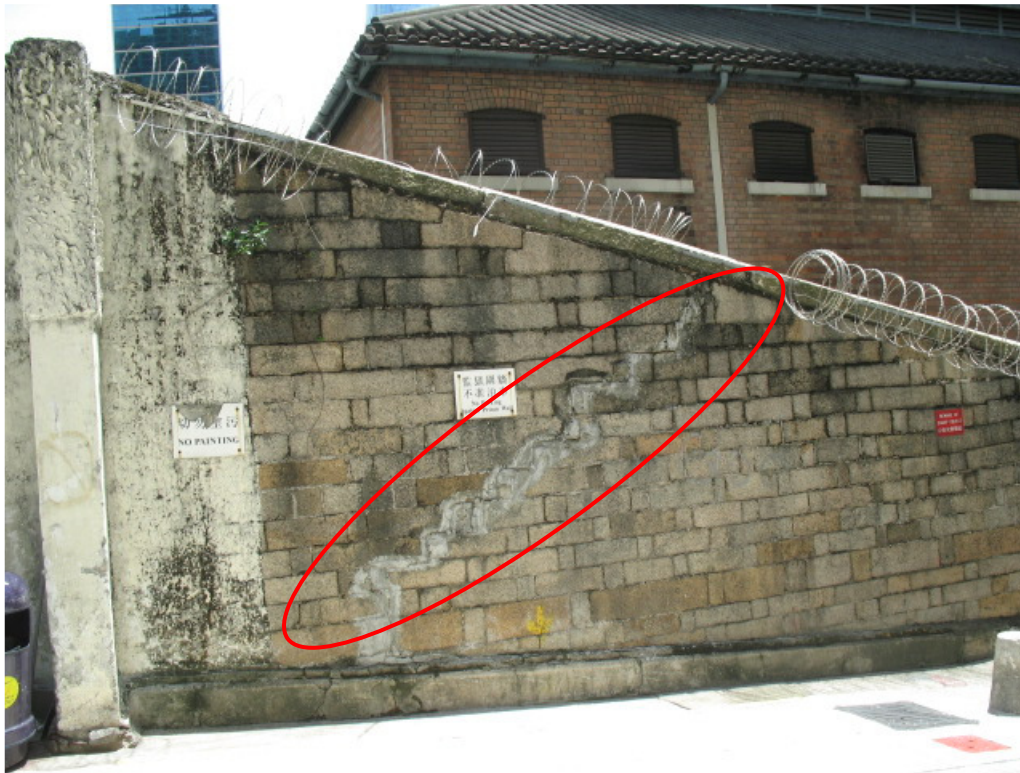
Photo ex 27a – Crack is found on the wall.
