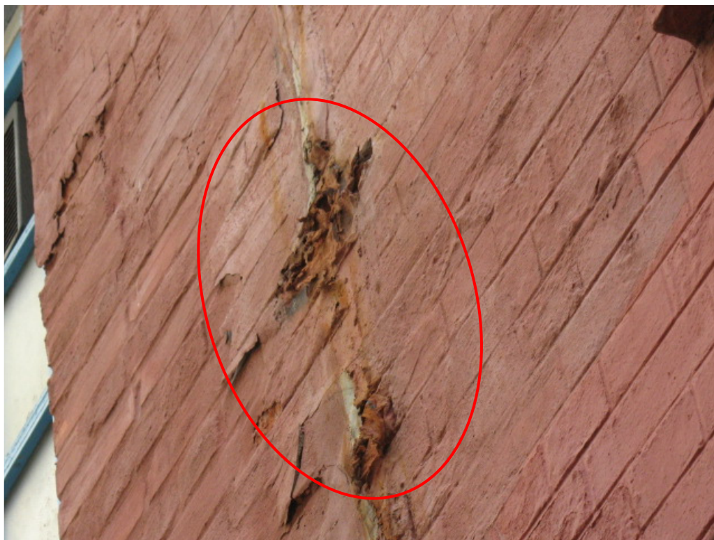
Photo ex 09b – The wall is damaged.
