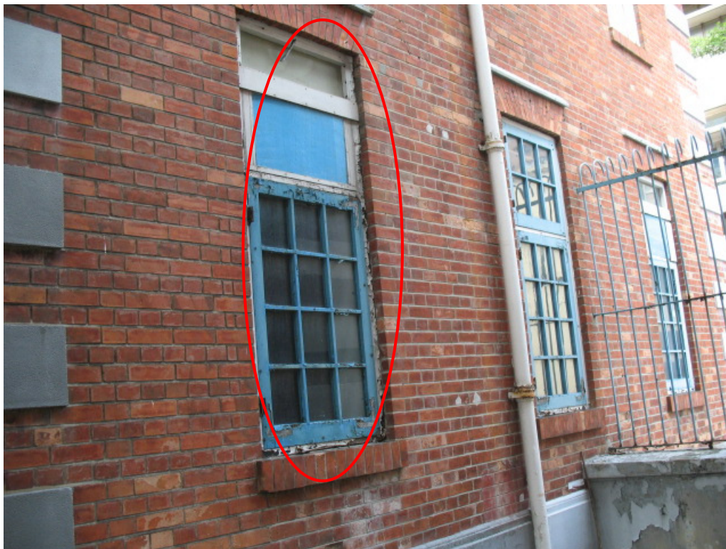
Photo ex 04a – The window frame is damaged.
