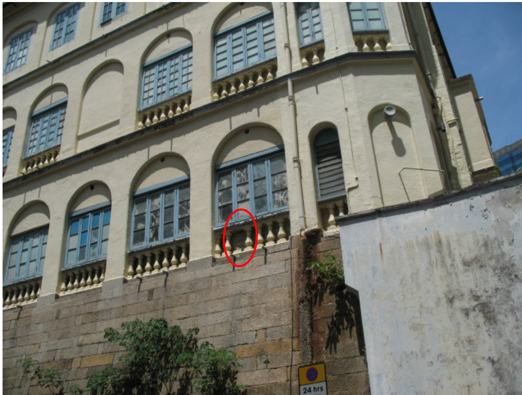
Photo ex 31a – One of the feature is missing.
