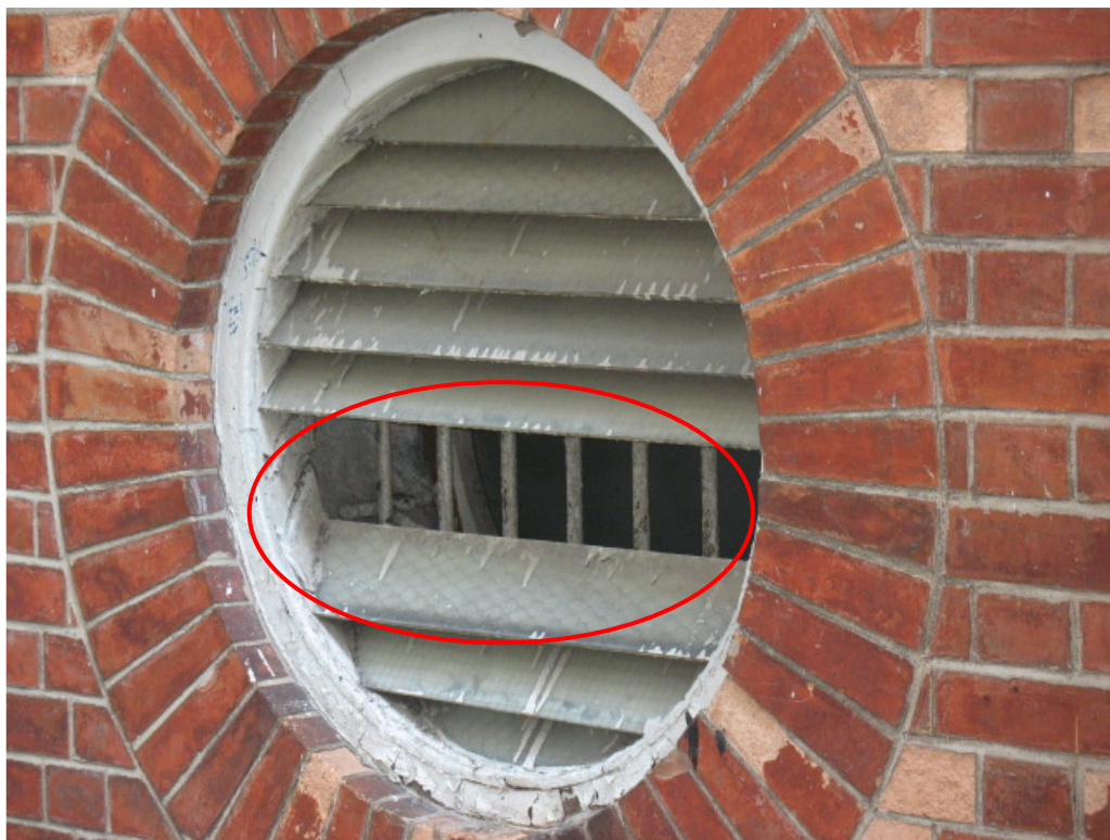
Photo ex 07b – The window is damaged.
