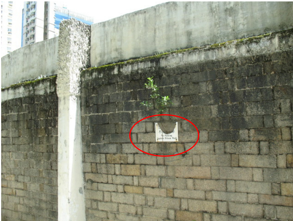
Photo ex 26a – The notice plaque is damaged.
