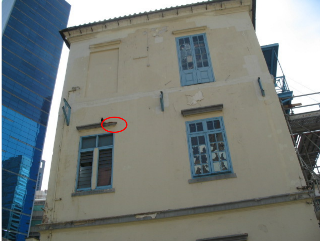
Photo ex 01a – The wall feature is chipped.
