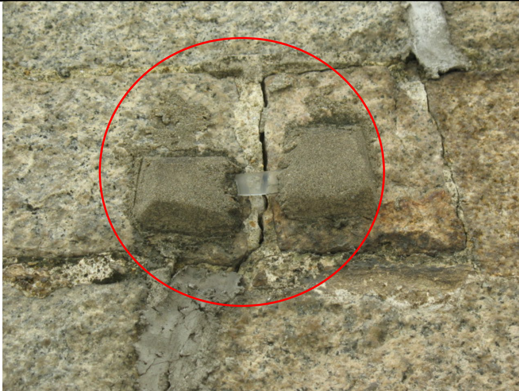
Photo ex 22f – Crack is found on the wall.
