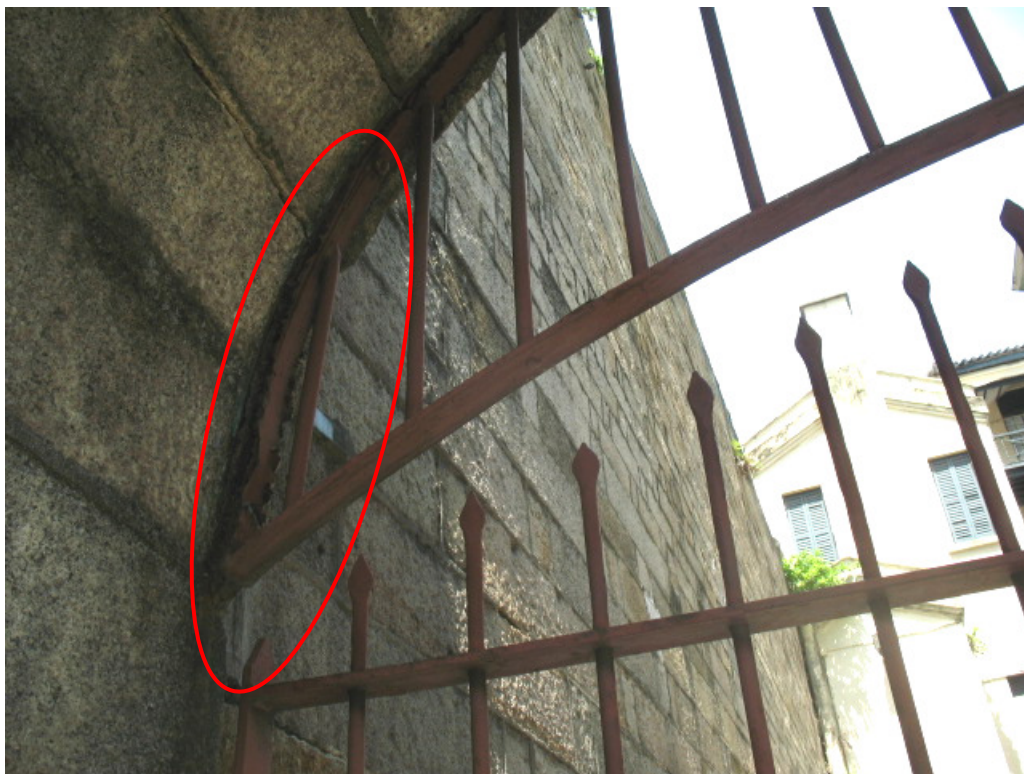
Photo ex 29b – Corrosion is found on the gate.
