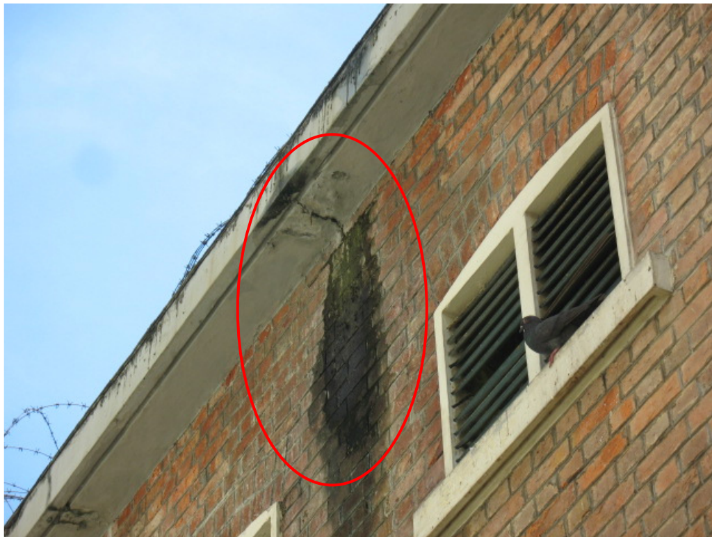
Photo ex 15b – Crack and water stain are found on the wall.
