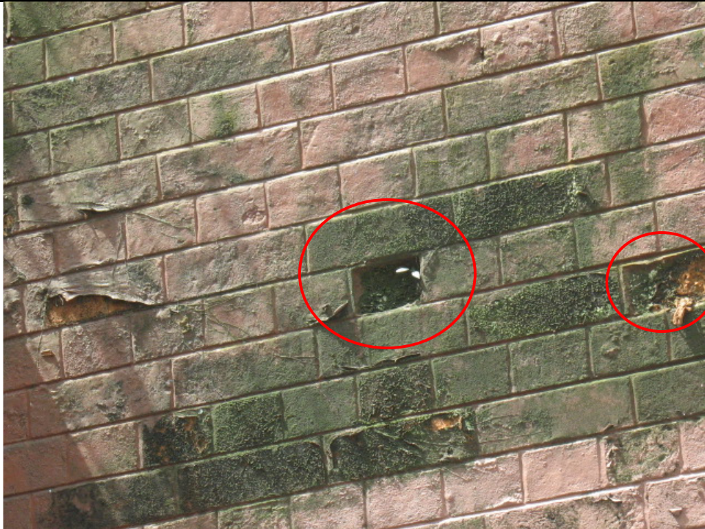
Photo ex 22b – The brickwork is damaged.
