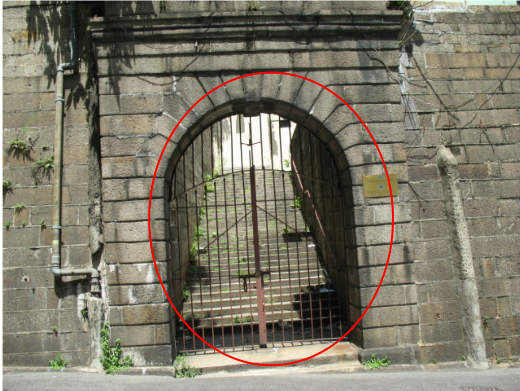
Photo ex 29a –Corrosion is found on the gate.
