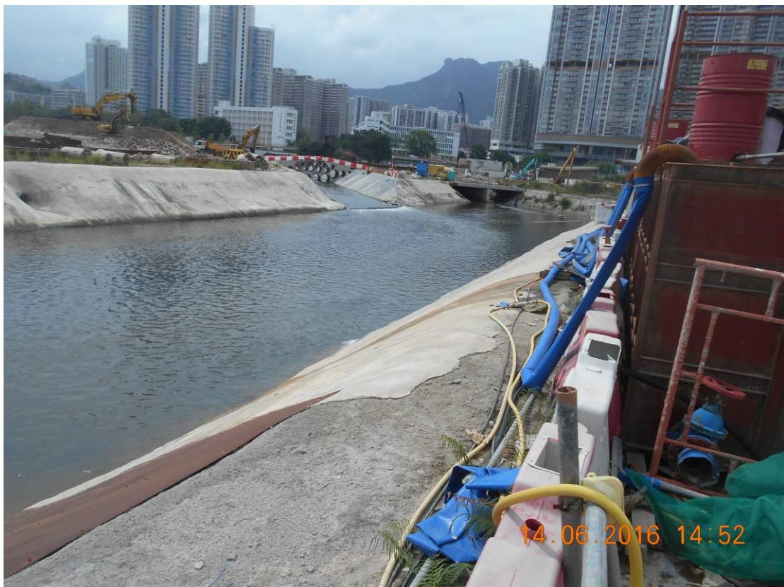
Fig.2 – Sedimentation tank was provided for desilting.
