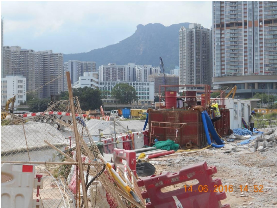
Fig.1 – Sedimentation tank was provided for desilting.
