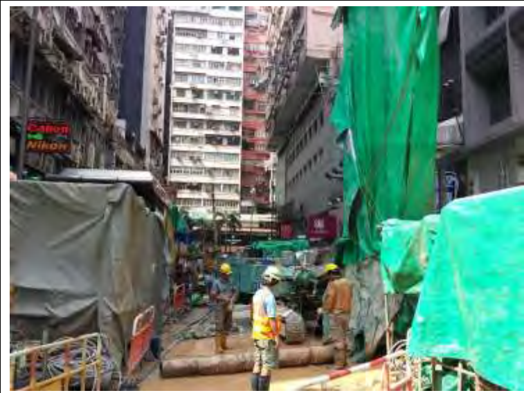
Air compressor (left) and drill rig (right) located near the main entrance was fully enclosed by multi layers noise insulation mat and tarpaulin respectively.
