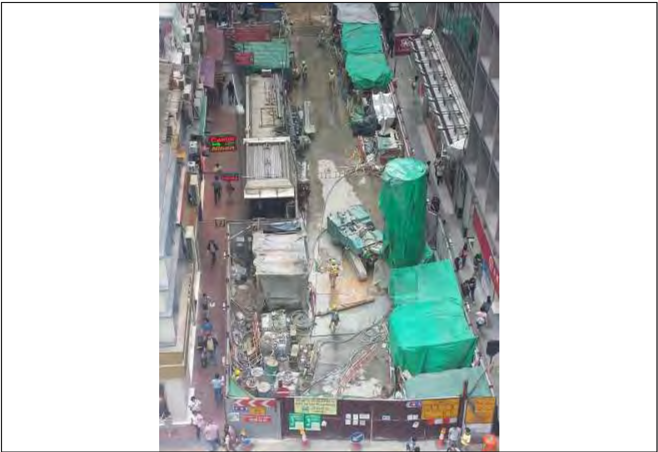
Site hoarding had been laid with noise insulation mat along the site boundary.
