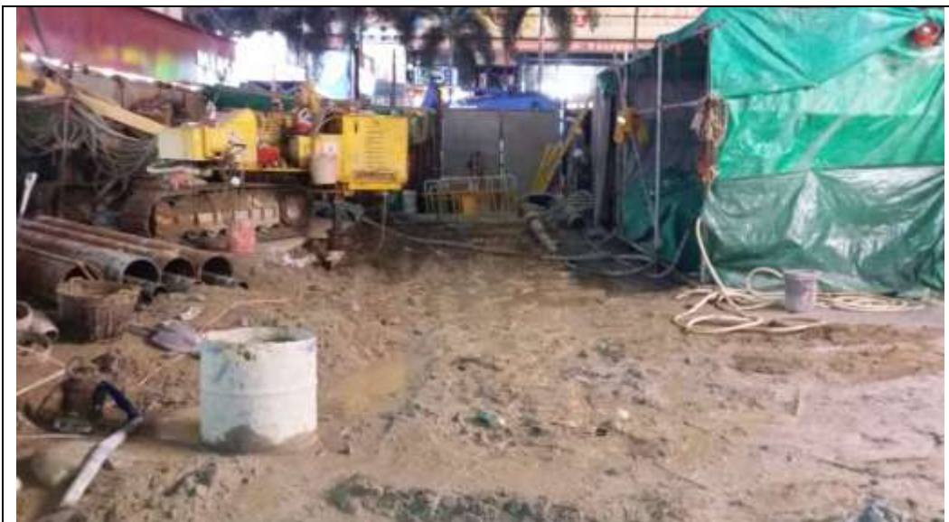
All PME's had finished mobilization and parked on site before 19:00hr. (Photo provided by main contractor which taken on 6 Nov 2014 18:56hr.)
