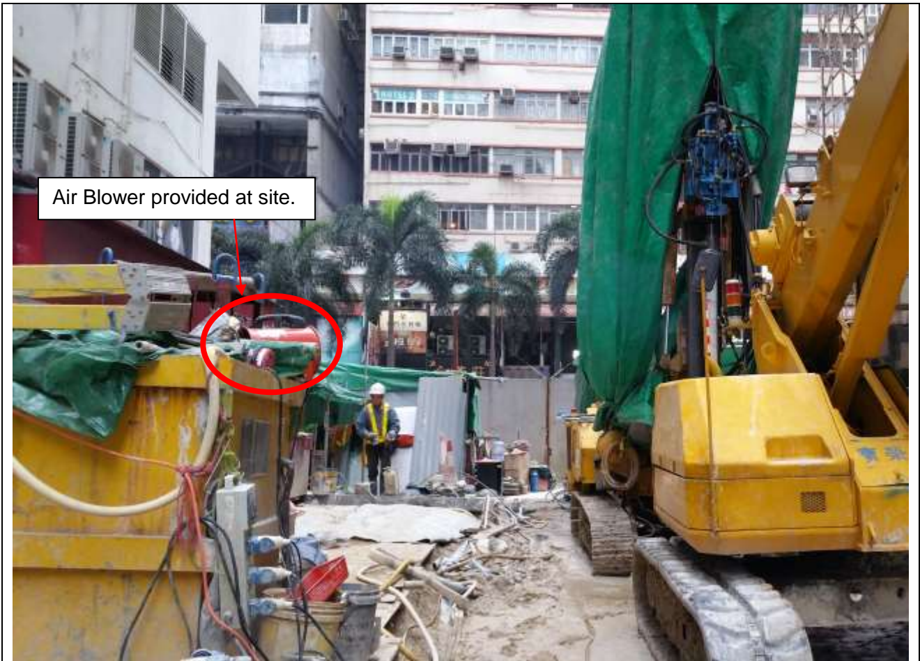
Blower was used for ventilation purpose during engine start-up at site. (Photo provided by the Contractor on 07 February 2015).
