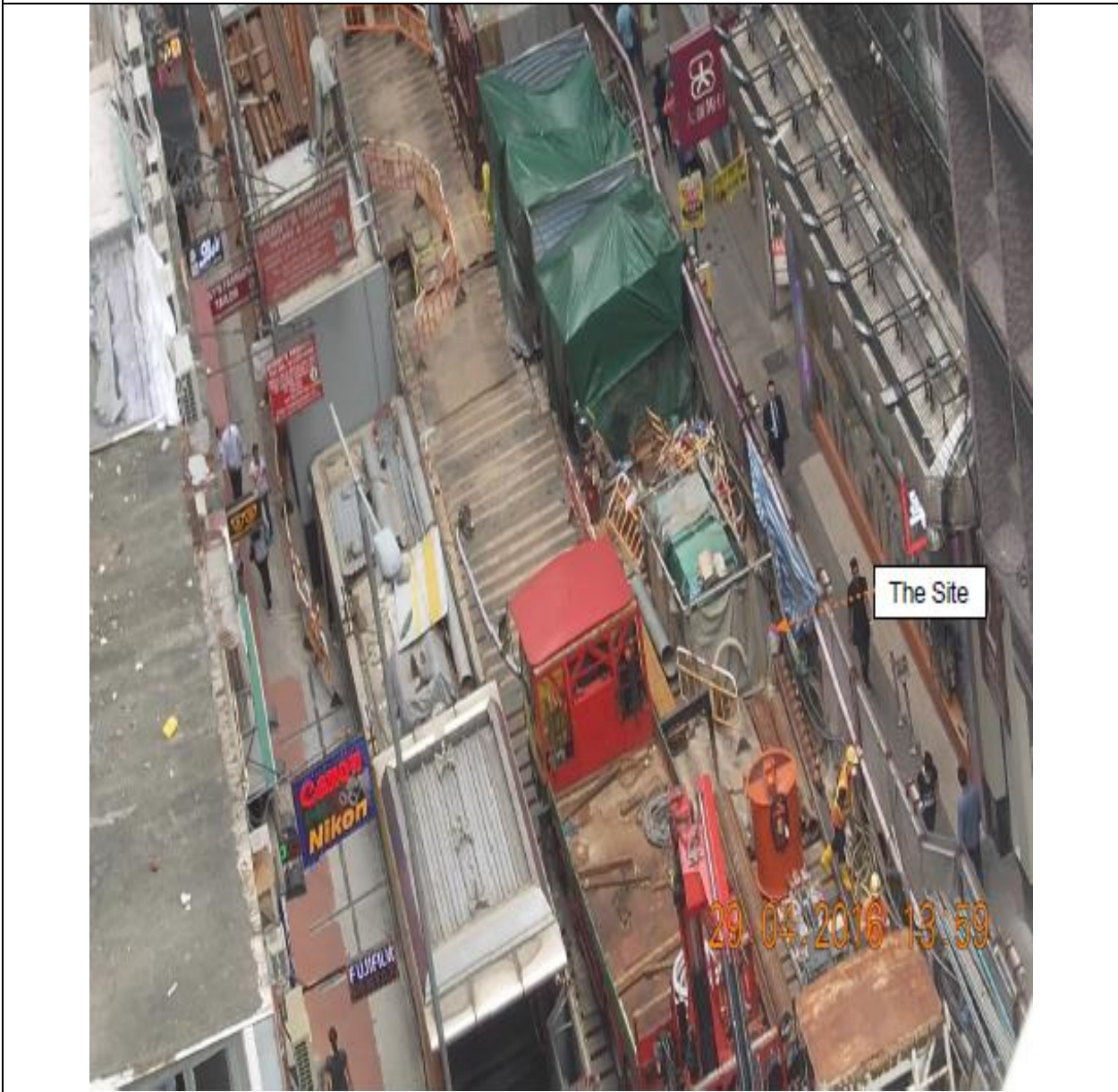
Photo 8 Free of construction dust within the site as a result of implementation of effective dust suppression measures
