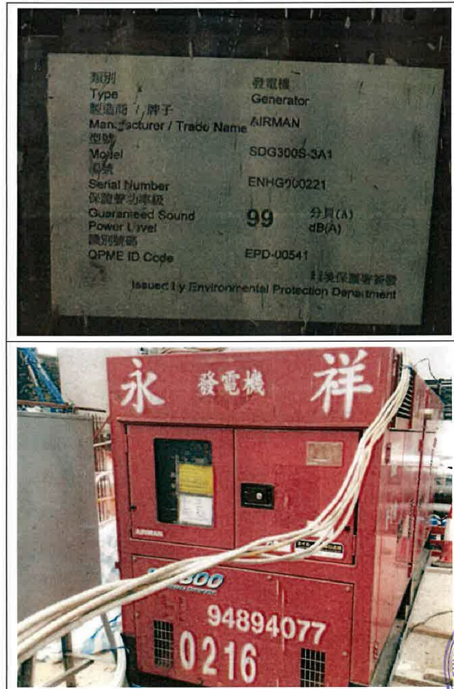
Generator, with Quality Powered Mechanical Equipment Label showing the Sound Power Level of \leq 99 dB(A)
