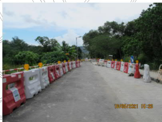
PHOTO 1378: HA WAN TSUEN EAST ROAD UNDER ROAD IMPROVEMENT WORKS (PHOTO TAKEN: 18 MAY 2021)
