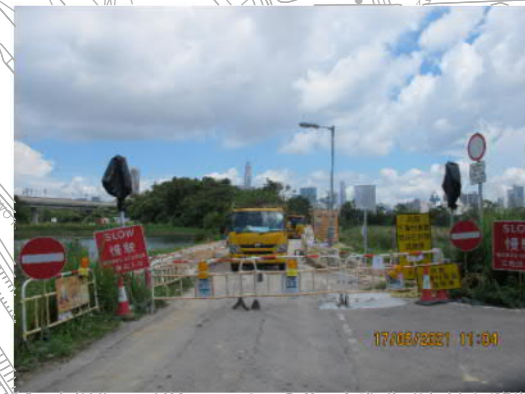
PHOTO 7393: HA WAN TSUEN EAST ROAD UNDER ROAD IMPROVEMENT WORKS (PHOTO TAKEN: 17 MAY 2021)
