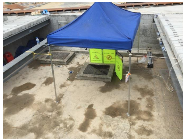
Photo 4 - Some litter and debris were observed on the Project site during site inspection on 26 May 2016.
