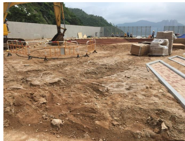
Photo 2 - The drainage system for the CU site (within which the APG Project is located) had loose and exposed soil during the site inspection on 26 May 2016. The CU site manager confirmed that site runoff from CU site would drain away from APG BMH area and therefore the site runoff from CU site was not considered an issue for the APG BMH (see also Annex A).
