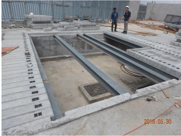
Photo 5 - Land works were completed and BMH Manhole was closed during the Project site inspection on 30 May 2016.
