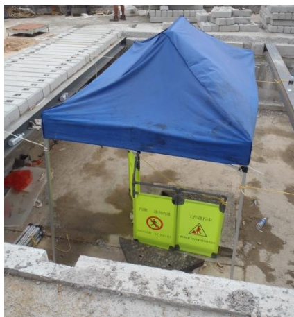
Photo 1 - The BMH Manhole Cover was open for the Project works to occur/caution was taken during the site inspection on 26 May 2016.
