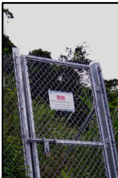
Photo 3 – Currently Situation of Protective Fencing and Warning Sign
