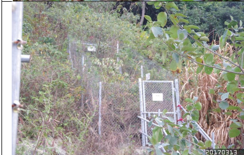
Photo 3 – Currently Situation of Protective Fencing and Warning Sign
