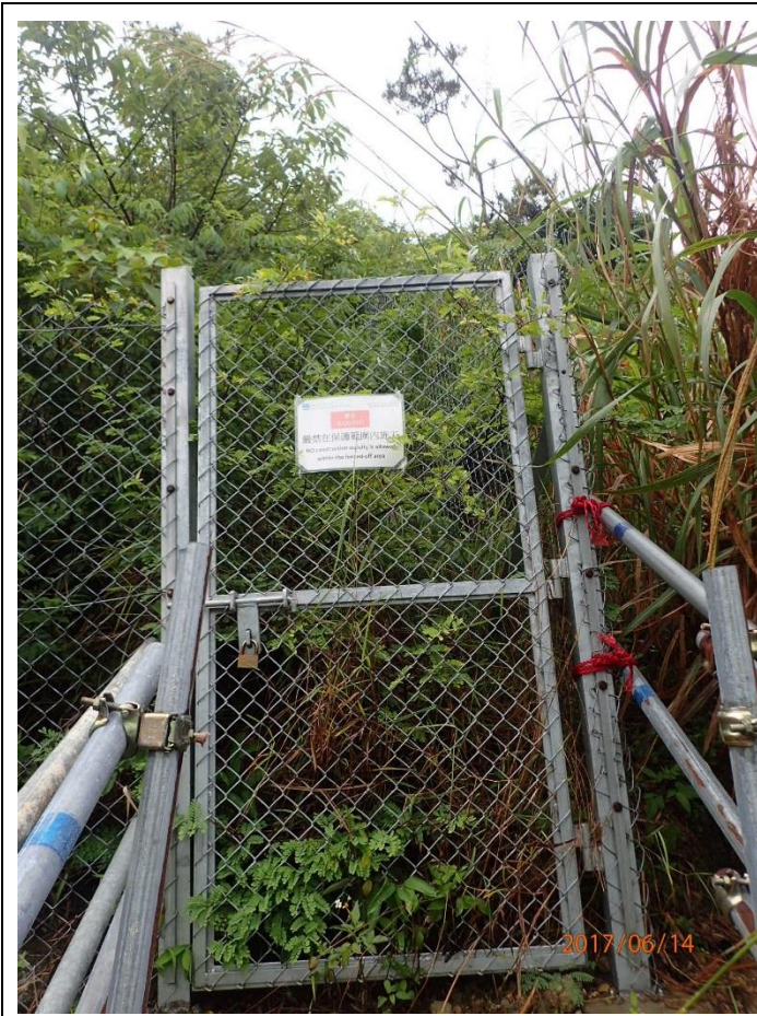
Photo 3 – Currently situation of fencing and warning sign
