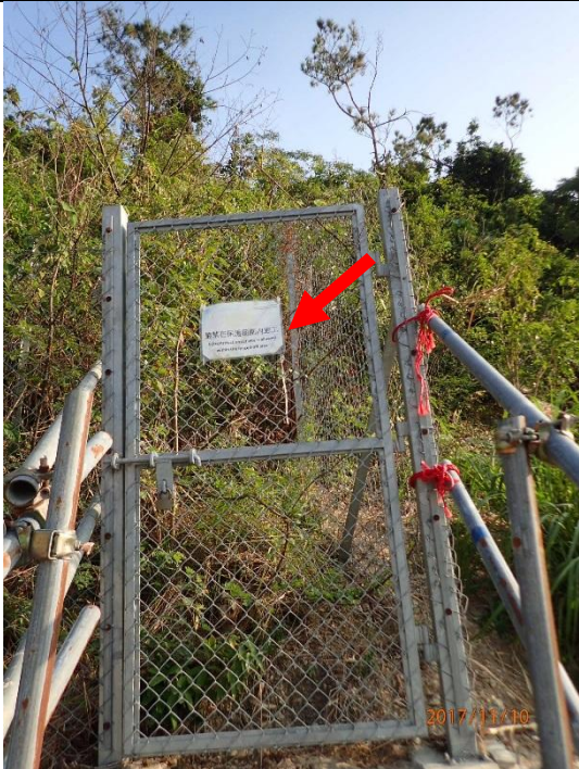
Photo 2 – Current situation of fencing and warning sign
