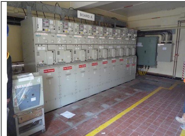
Photo 7 – Switch Panel Room at the substation
