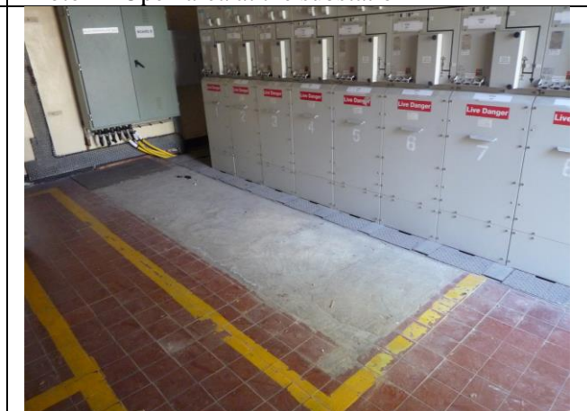
Photo 6 – Switch Panel Room at the substation
