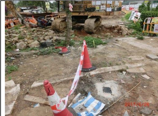
Installed groundwater well
