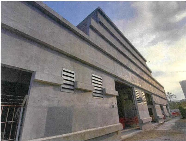
Photo 3 –Silencer installed at the outlet of extraction fans (View A)
