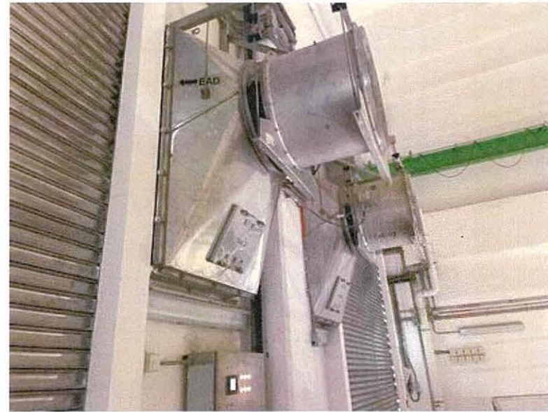
Photo 2 – Extraction Fan (Inside)
