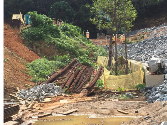
Description: Stockpile of construction materials should be avoided at the protection zone and protective fence for Aquilaria sinensis should be properly erected and maintained.
