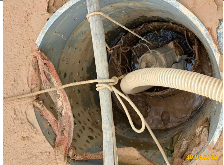
Submersible pump in place and dewatering was carrying out to drain away the collected surface runoff when it was raining
