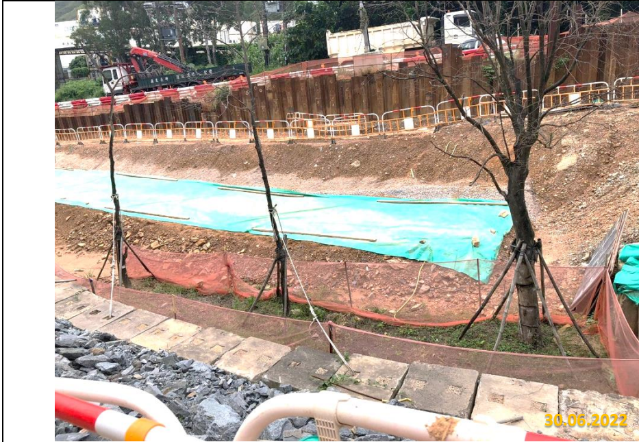
Formation of ditch to divert the surface runoff into water collection point
