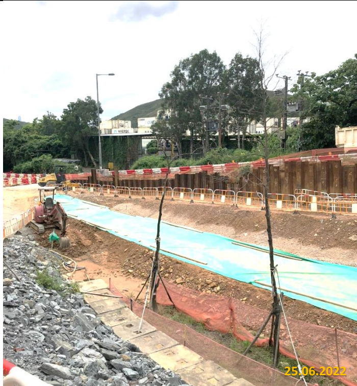
Formation of ditch to divert the surface runoff into water collection point
