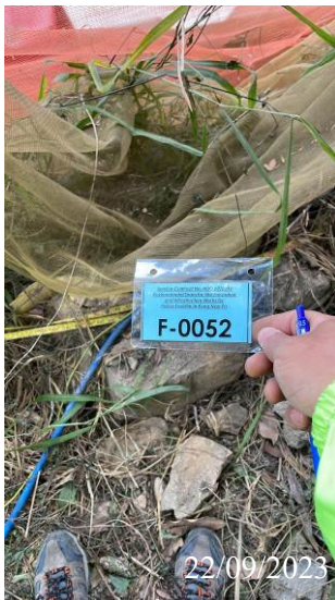
F-0052 was found collapsed in the reporting month after typhoon / adverse weather condition.
