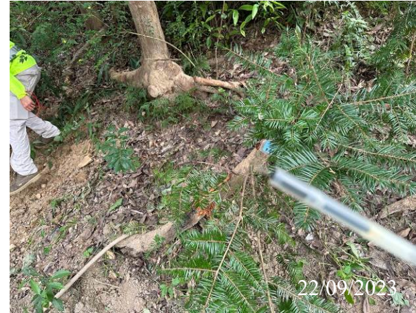
F-0051 was found collapsed in the reporting month after typhoon / adverse weather condition.
