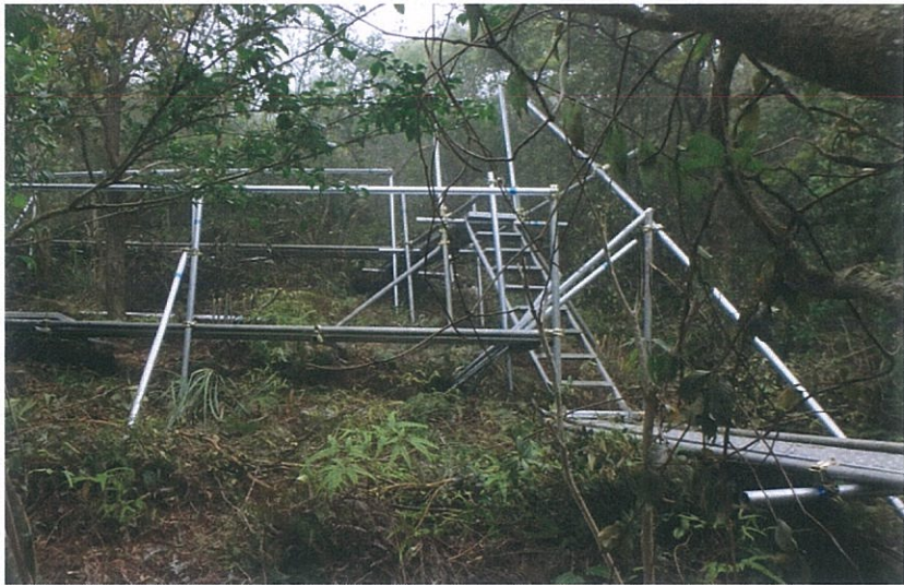
Plate 1. Vegetation clearance was kept at minimum for building temporary access to the transplantation receptor site.
