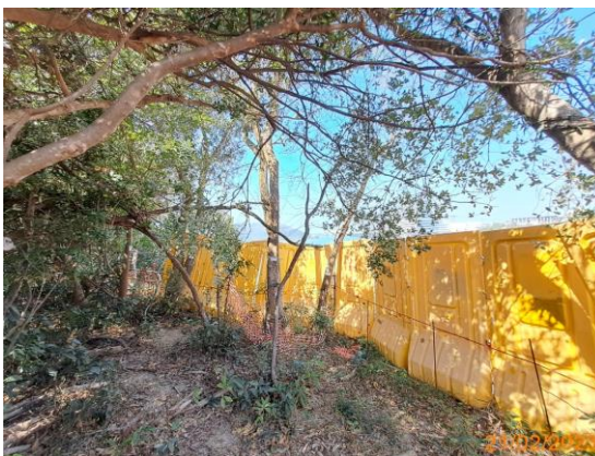
6: Temporary protective fencing for U041, U042 and U043 (1)
