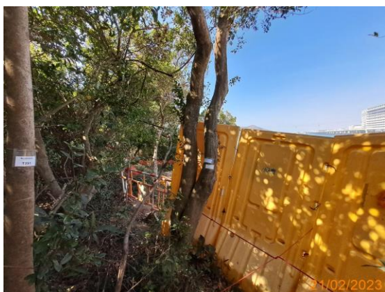
7: Temporary protective fencing for U041, U042 and U043 (2)
