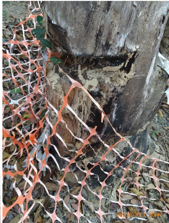
4: U041_Old termite track
