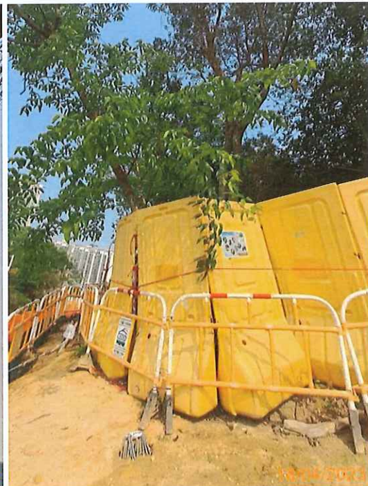
8: Temporary protective fencing for U041, U042 and U043
