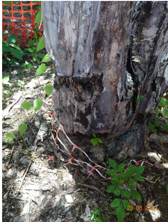
8: U041_Wood damaged by termite
